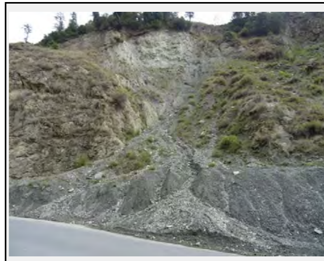
Part of the slope is highly eroded and shows multiple gullies
