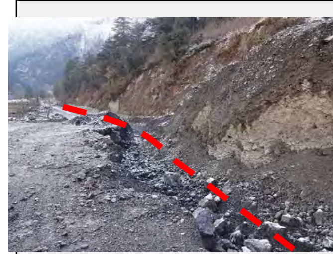
Road condition: Existing road is still buried 5m under the talus deposits.
