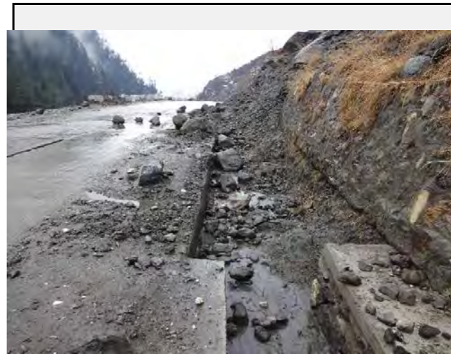
Existing countermeasures / anomalies: Some part of the water canal are filled with the debris.
