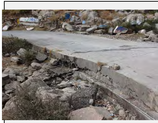
Existing countermeasures : Three pipe culvert are installed under the causeway.
