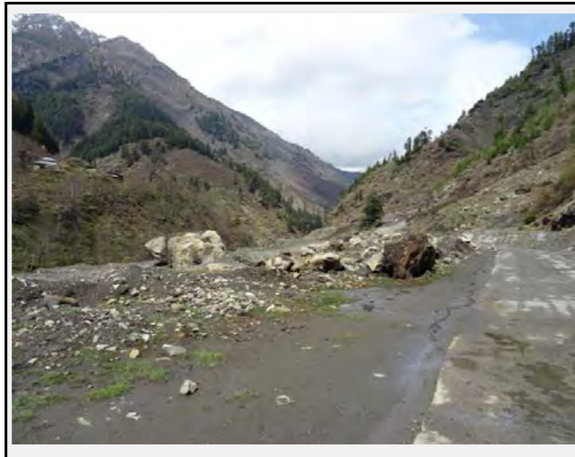
There is evidence of rock falls in the past that have been pushed to the valley side to clear the road
