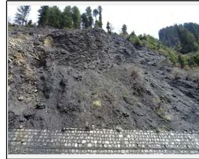
The debris and rocks detached from the highly weathered base rock surpass the retaining wall and fall on top of the road
