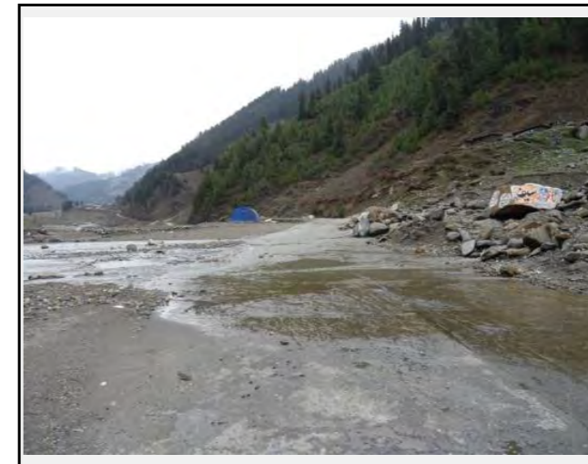
The road is flooded and partially covered by debris
