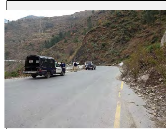
Road condition: No anomalies or damages was confirmed on the road though there was a small portion of talus deposit observed at the shoulder of the road.
