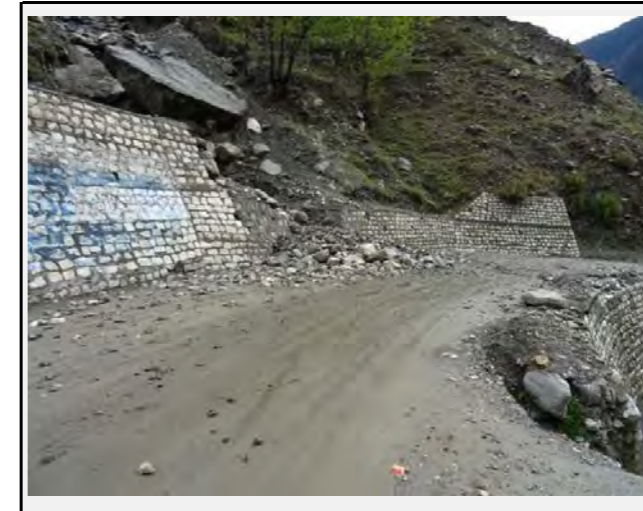
Road condition: there is mud and debris on the road and the road surface is damaged considerably
