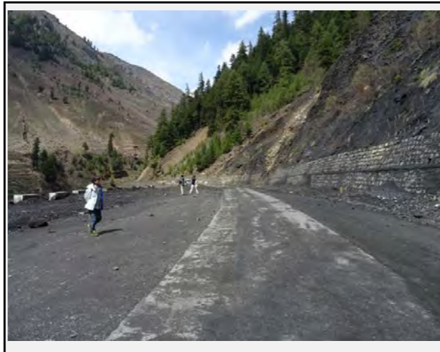
Condition of the road: the road needs to be cleared regularly due to constant collapse of the slope. The debris are removed to the valley side of the road.
