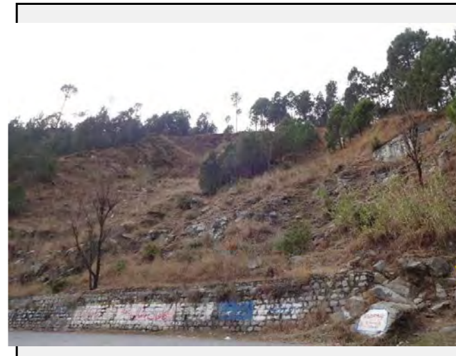
Others: Trace of the slope failure at the side of the stream. Retaining wall is constructed at the toe of the slope. However, the slope is covered with vegetation and seems stable.
