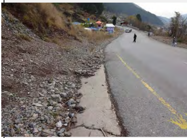
Existing countermeasures: The waterway is filled mostly by the talus.
