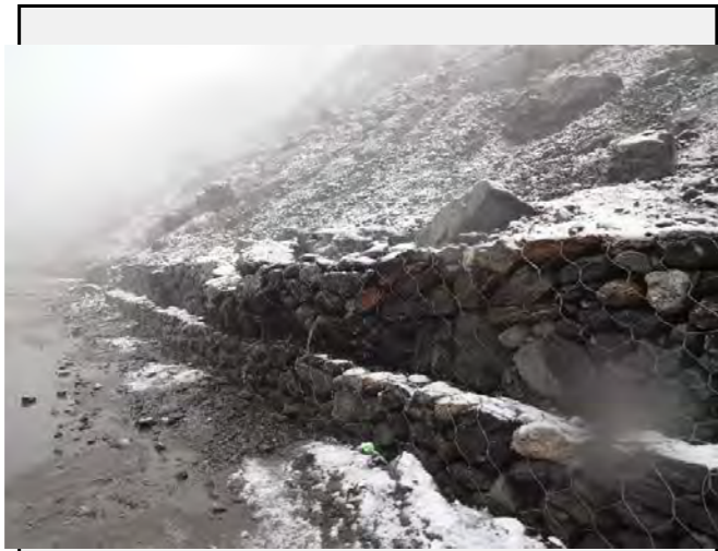
Existing countermeasures / anomalies: Several damages on the gabions was confirmed due to overload of the deposit.
