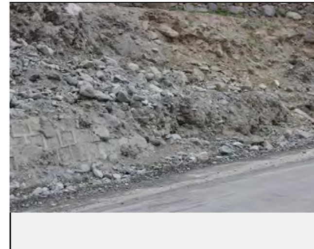
Existing countermeasures / anomalies: Retaining Wall has been constructed along the Debris Flow
