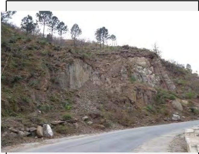
Mountain side: Both slope failure and rock fall was observed at this site.
