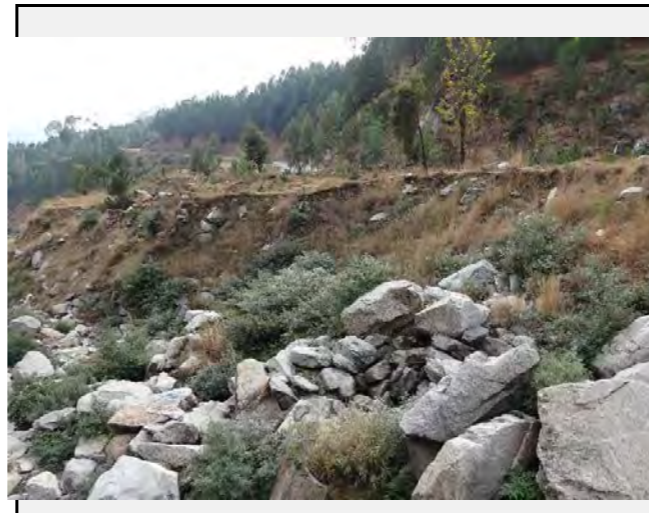
Existing anomalies: Some trace of the slope failure was observed on the valley side of the road.
