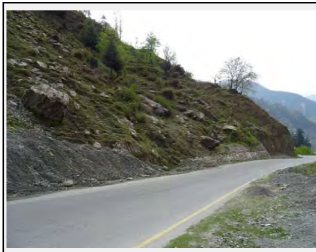
Existing countermeasures: Retaining walls are constructed partially on the mountain side. They are partially damaged by the slide
