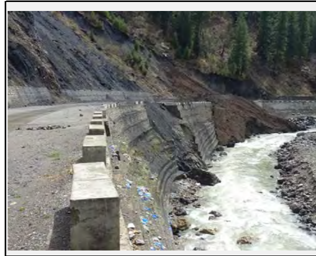
The valley side of the road is located in the outer curve of a river but it is protected by a concrete wall
