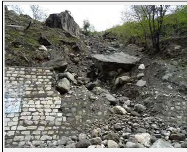
Existing countermeasures / anomalies: The exit of the retaining wall on the mountain side was re-shaped to allow the debris flow. However, this is resulting a steeper angle of the stream. The thickness of the sediment in the stream bed is around 2m
