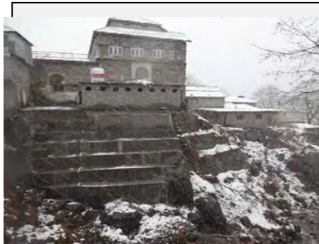
Existing countermeasures: Retaining wall is constructed on the both side of the bridge to protect the bank erosion.
