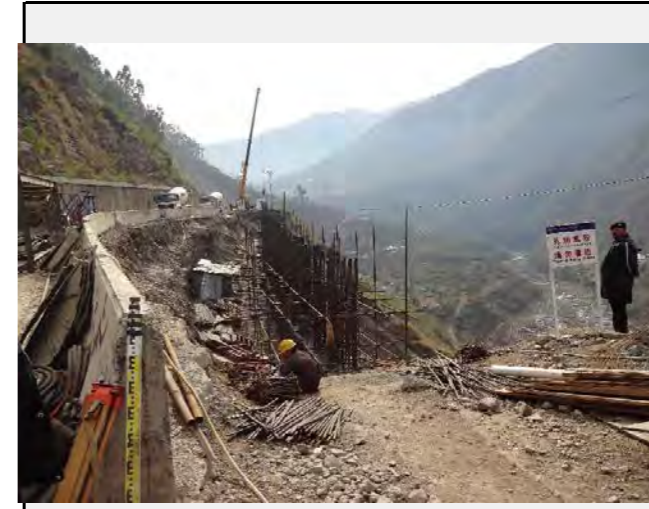
Road condition: Construction on shifting the road alignment to the valley side is being carried out by CPEC.
