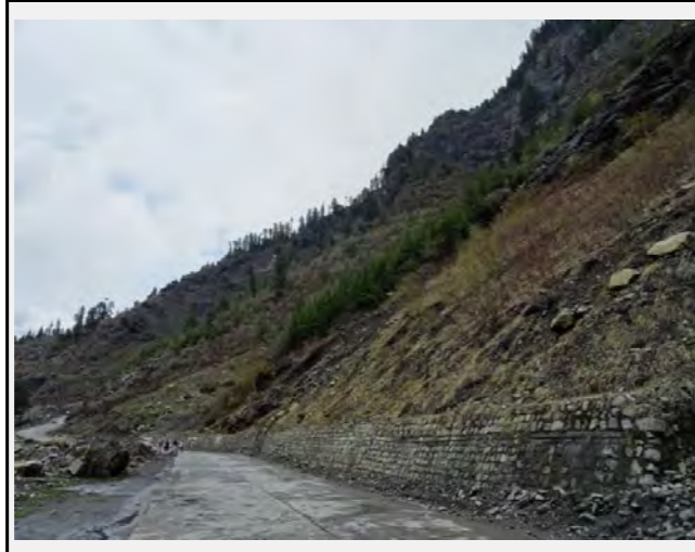
A vertical rock wall of approximately 250 m produces rock falls towards the road. The retaining wall has no effect as a countermeasure for rock falls
