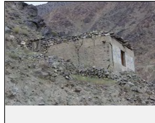
Existing countermeasures / anomalies: No Counter Measure. House has been damaged along the Debris Flow
