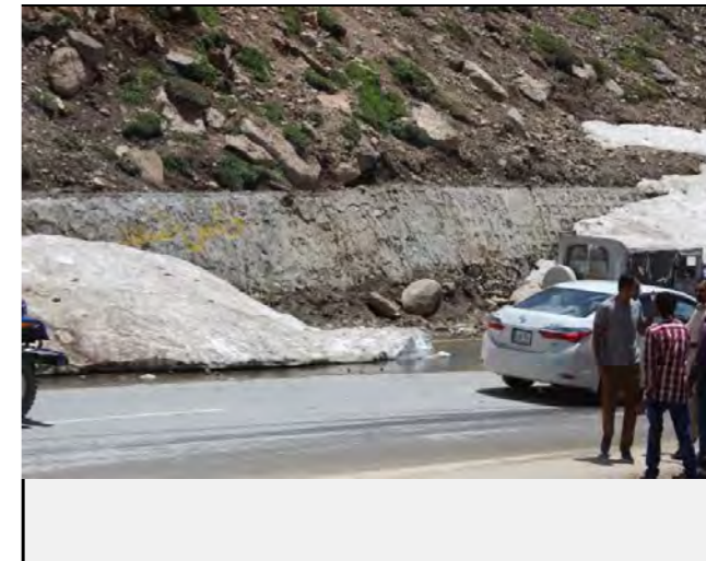
Existing countermeasures / anomalies: Retaining wall has been constructed along the Debris Flow
