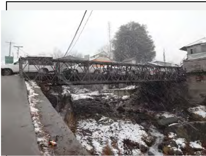
Existing countermeasures: The height of the bridge from the stream bed seems have enough capacity for debris flows at present.
