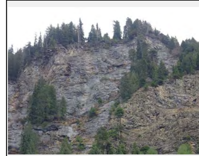
The vertical rock wall that produces the falls seems to have significant fractures
