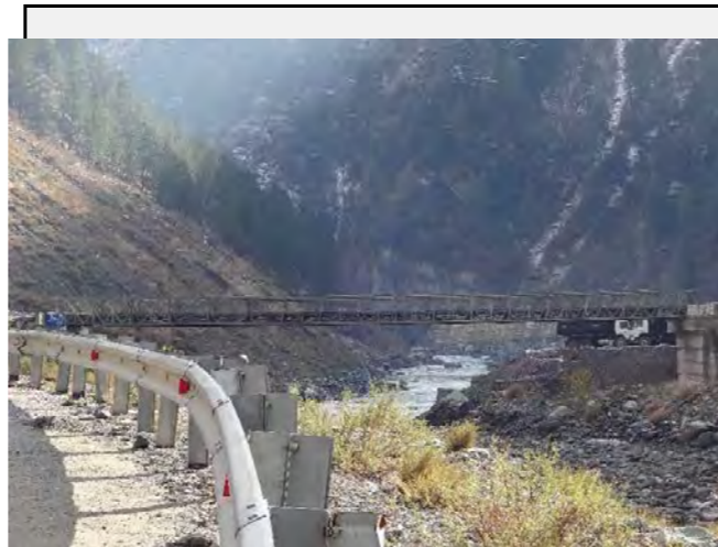
Existing countermeasures: Bailey bridge is used as temporary on the bypass road.
