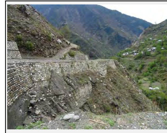
Possible countermeasures: a bridge can be constructed in the valley side of the road avoiding the debris flow stream.
