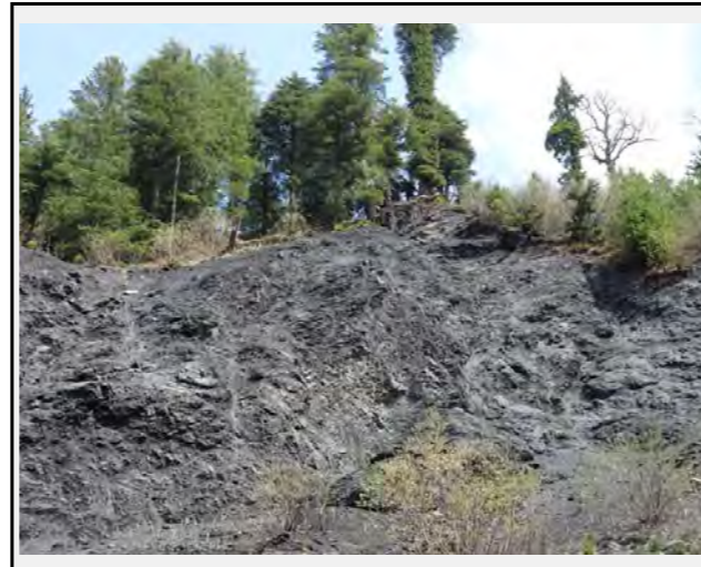
Outcrops of the base rock can be identified throughout the slope. The outcrops are highly weathered and fractured.
