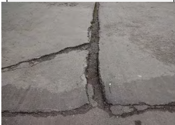
Existing anomalies: Cracks (20cm) was confirmed on the replaced portion of the road.
