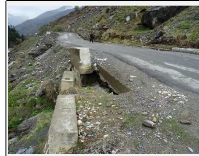
Road condition: Two area of the road subsidence was confirmed. There might be a cavity underneath the road.
