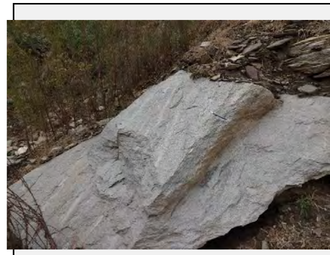
Existing anomalies: The size of the fallen rock is large enough to damage the road or cars.
