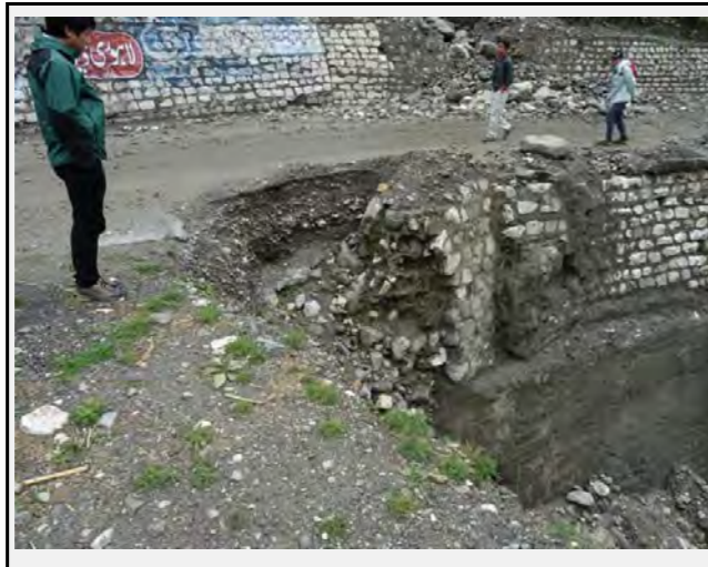
Existing countermeasures / anomalies: small damage (2m) of the retaining wall on the shoulder of the road (valley side) due to the debris flow.
