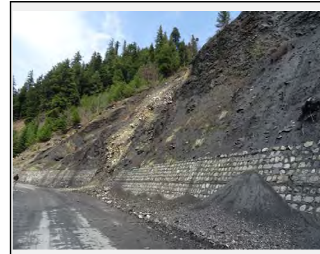
In some sections the retaining wall is damaged and the debris reach the road directly.
