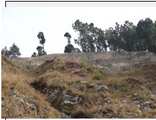
Existing countermeasures : Shotcrete was undertaken by FWO on the head of the slope to minimize the surface erosion.
