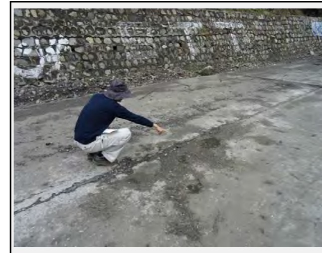
The rock falls cause damage on the road bed forming pot holes
