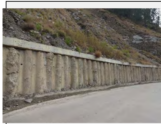
Existing countermeasures: Retaining wall (with piling) constructed at the toe of the slope.
