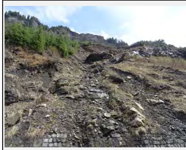
Fallen rocks that have not reached the road but may collapse and fall again can be identified throughout the slope
