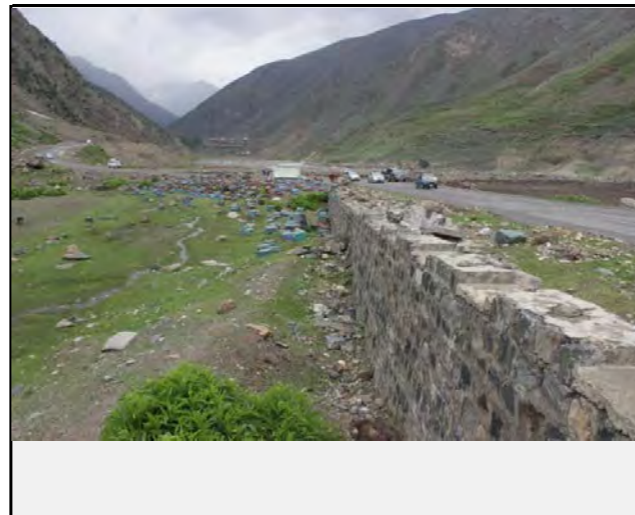
Existing countermeasures / anomalies
