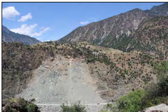
Full view of the landslide
