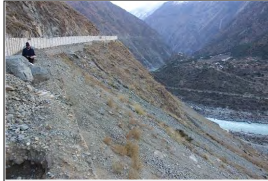
View of landslide on Valley side:
