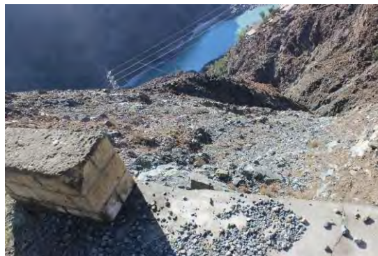
View of landslide on Valley side:
