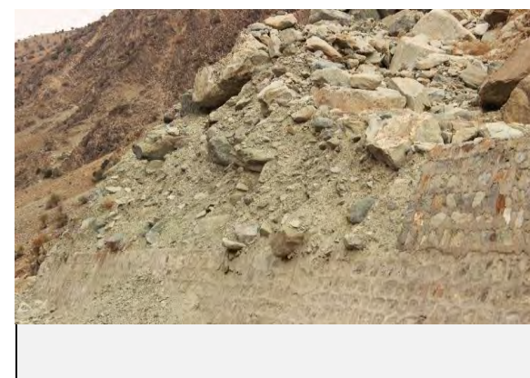
View of fallen blocks
