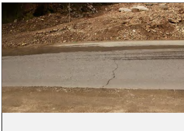
The crack on road has been observed
