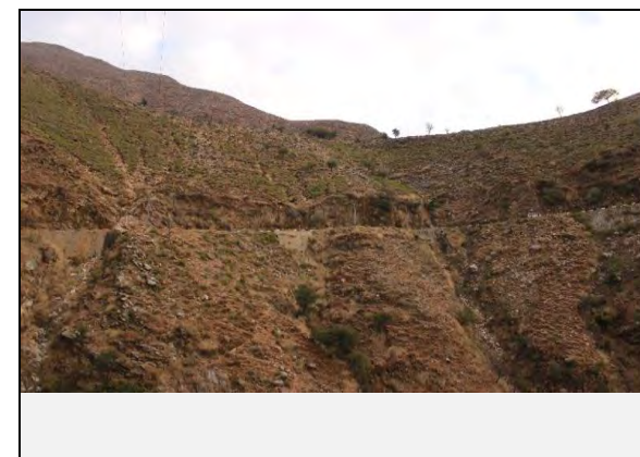
Close View of slope failure
