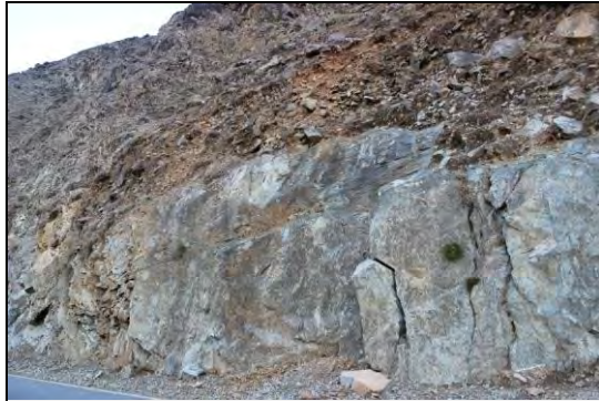
Full view of the landslide
