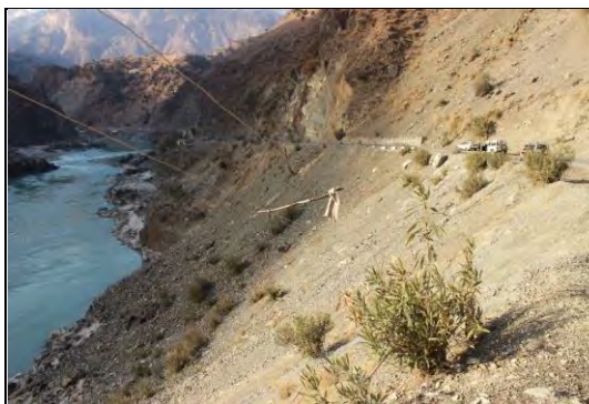
View of landslide on Valley side:
