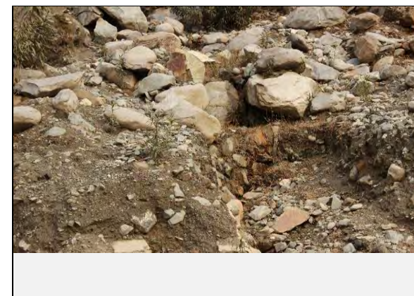
View of fallen blocks along slope failure
