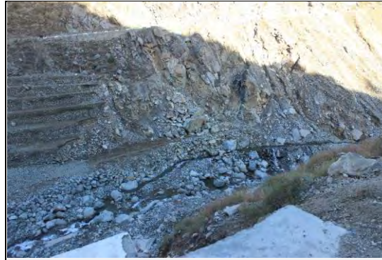
View of landslide on Valley side:
