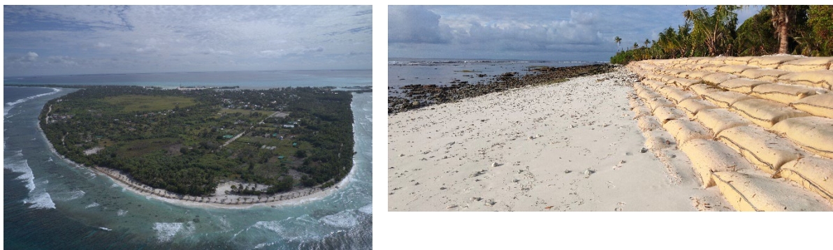
Figure 4.2.7 Sandbag Revetment under Construction by MNPFI as an Emergency Project (as of September 2022)
