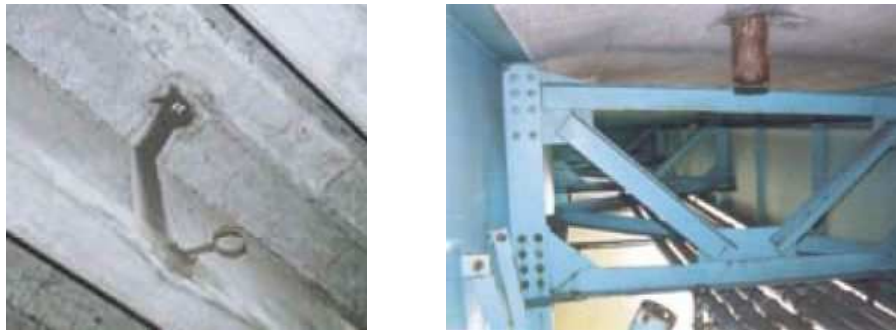
Figure 4.2 Example of Water Leakage (missing drainage pipes)
