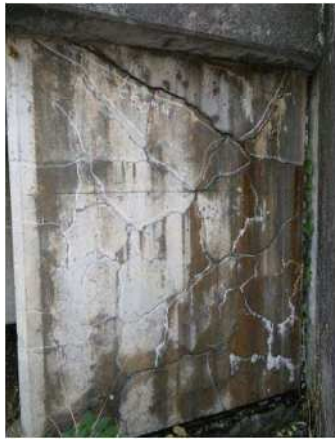
(Crack caused by ASR)
