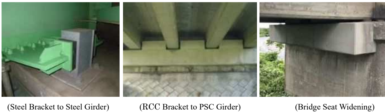
Figure 6.32 Example of Bridge Fall Prevention Device (Compression Force) and Bridge Seat Widening
