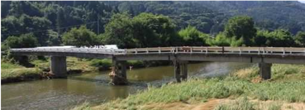
Figure 5.4 Example of Settlement/Inclination of Substructure which requires Detailed Observation
