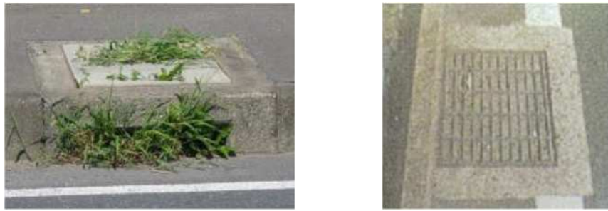
Figure 4.1 Example of clogging of drainage basin
