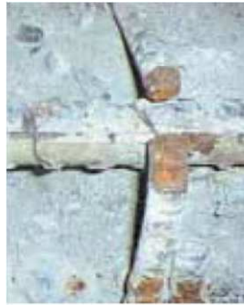
(Rebar torn by ASR)
