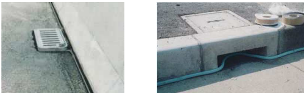
Figure 6.37 Example of Drain Pipe and Drain Basin
