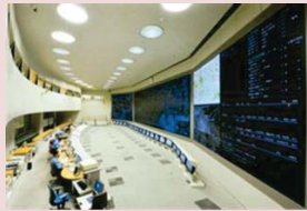
Traffic Management System
