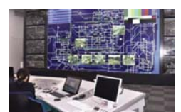
Traffic Control Center
