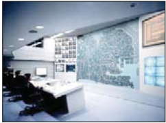
Advanced Traffic Management System
