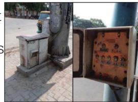
Existing signal controller box without key in Bengaluru city in India
