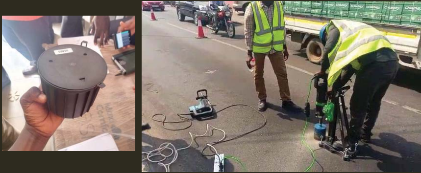
Installation of magneto detector in the road for detecting vehicular volumes, speeds and queue lengths
