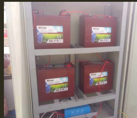
Battery for power back up for traffic lights
