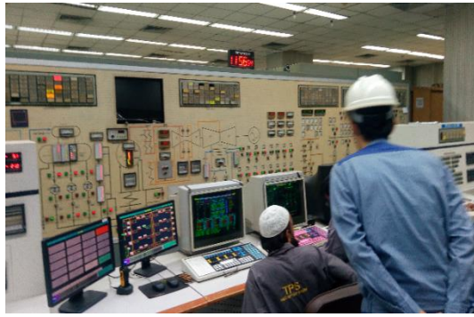
Site visit to Muzaffargarh TPS (2)
