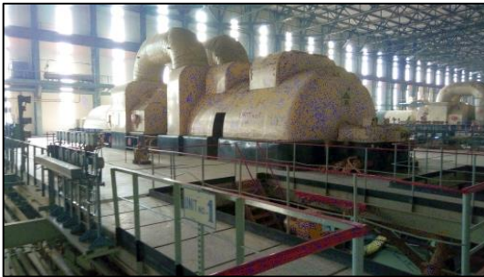
Site visit to Muzaffargarh TPS (1)
