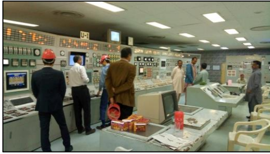
Site visit to Jamshoro TPS (1)
