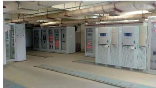
Site visit to Guddu TPS (6)
