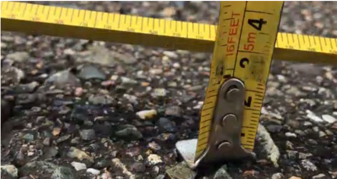
Figure 4.19 Rutting of Taxiway B
