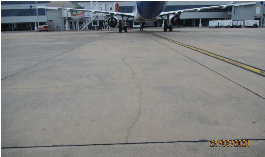
Figure 4.24 Cracks in Main Gear Position
