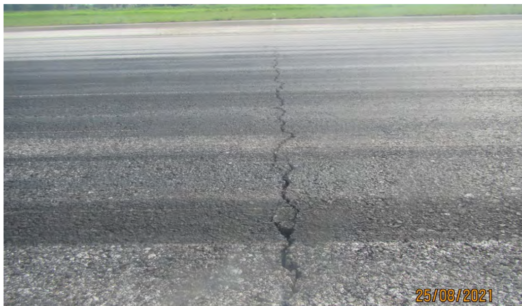
Figure 4.15 Example of Reflection Cracks on Runway
