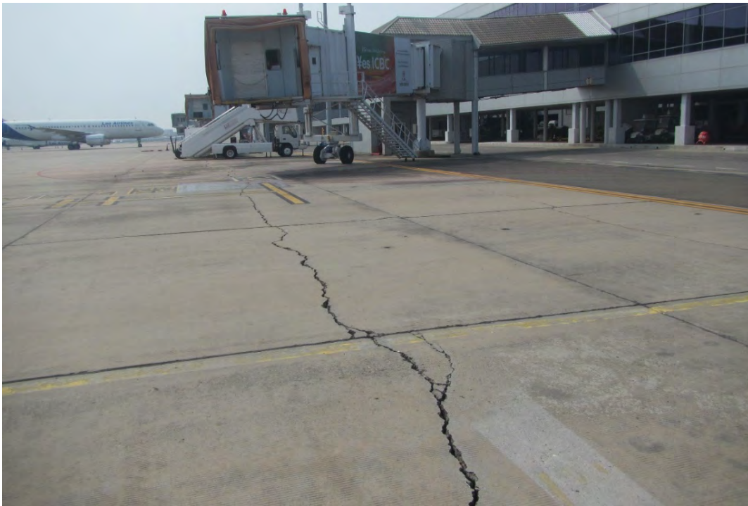
Figure 4.23 Apron Cracks in front of the International Passenger Terminal
