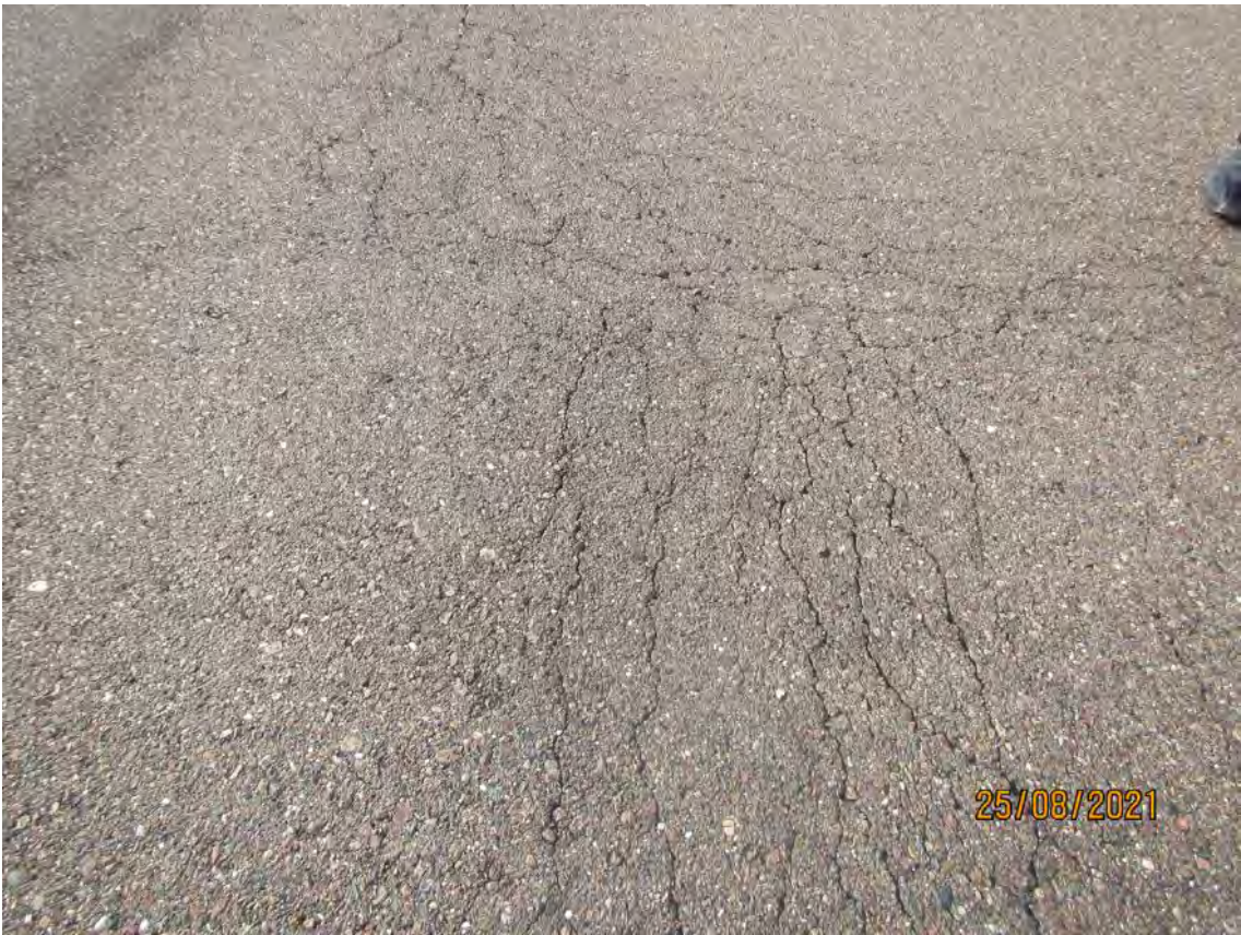
Figure 4.20 Alligator Cracks on Taxiway T
