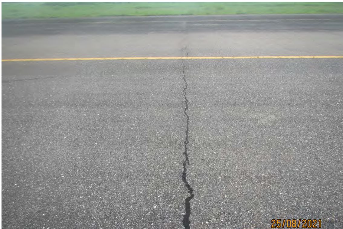
Figure 4.18 Reflection Cracks on Taxiway
