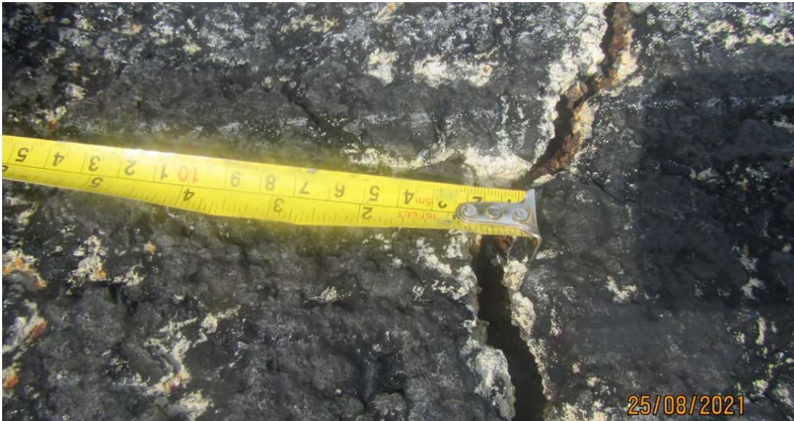
Figure 4.16 Close View of Crack on Runway
