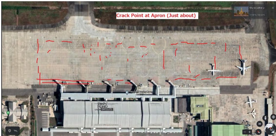
Figure 4 Severe Cracks in Apron
