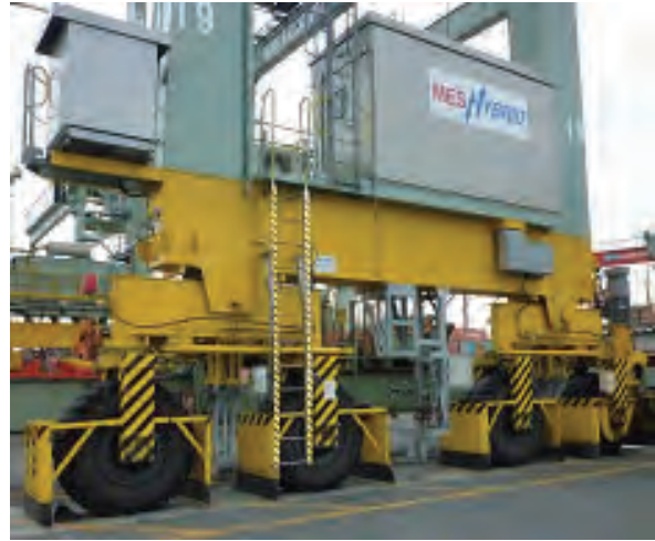
Gantry Travel Part (Electrical House Side)
