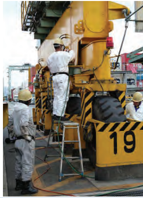
Clearance of Brake Pad of Steering Power Cylinder is checked and Brake units are cleaned by air-brush.
