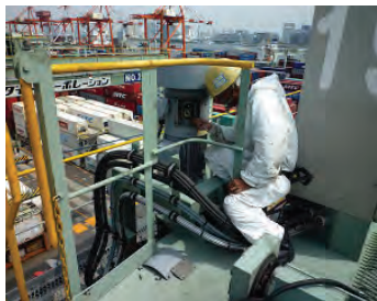
Clearance of Brake Pad of Trolley Traverse is checked and Brake unit is cleaned by air-brush
