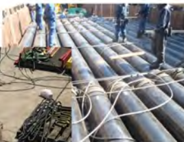
Need to prevent collapse
