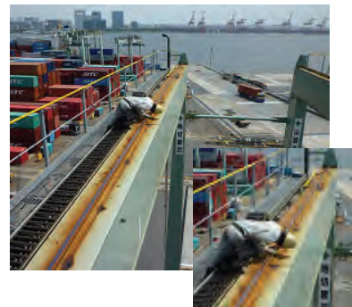
Confirmation of damage of the rail and crack in the welded line of traverse rail
