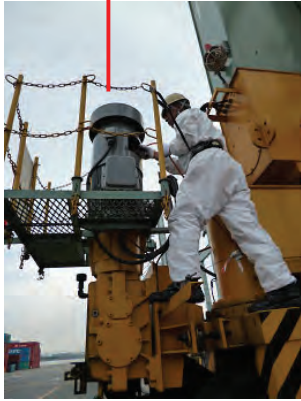
Clearance of pad of Travel Brake is checked and Brake units are cleaned by air-brush
