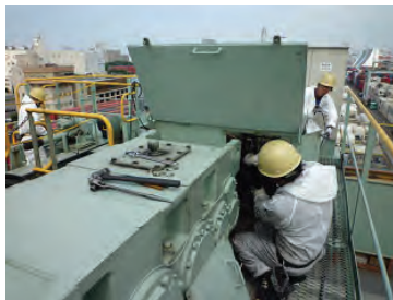
Clearance of Pad of Hoist Brake is checked and Brake unit is cleaned by air-brush
