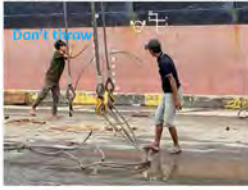
Dangerous wire works
