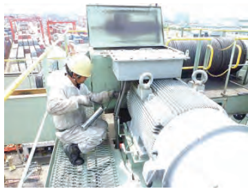
Refueling of grease to Disk Brake Coupling of Main Hoist Motor
