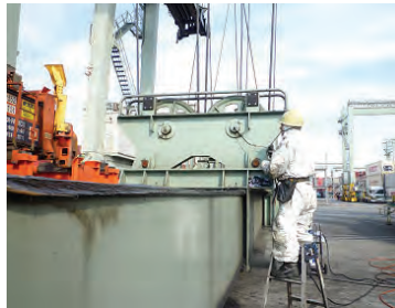
Refueling of grease to Sheave bearing
