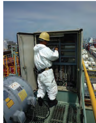
Operation of equipment such as a relay is checked.
