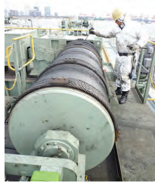
Confirmation of the damage of Hoist Ropes
