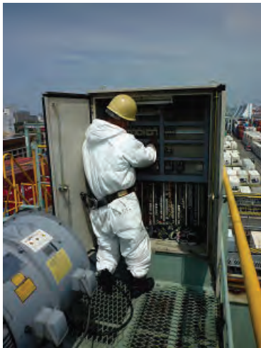
Electrical unit, module and other parts of Trolley Control Panel are cleaned by air-brush
