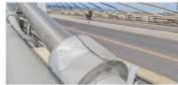
DEFORMED DAMPER DRUM
