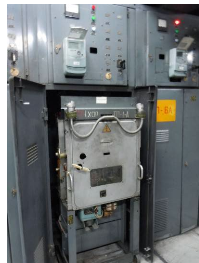
Cubicle of Russian Manufacturer
