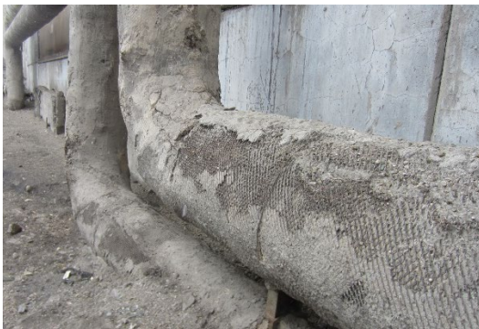
Hot Water Pipes with Deteriorated Insulation
