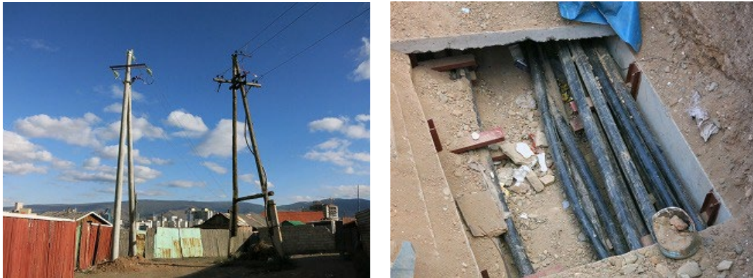
Figure 3-20 Distribution Lines (Overhead and Underground Lines)
