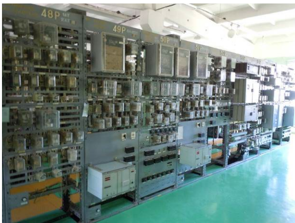
Relay Panels and Mechanical Relays
