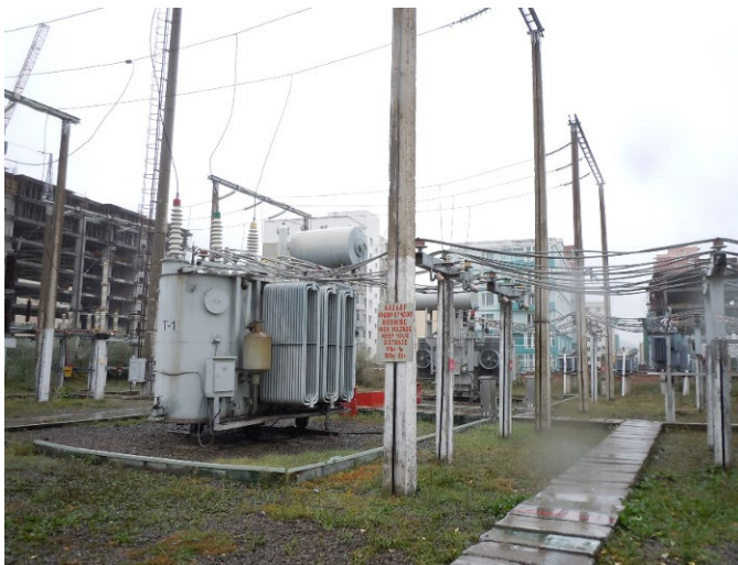
Transformer and Busbar of Existing Substation
