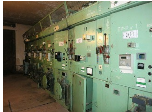
Switches in Switching Station
