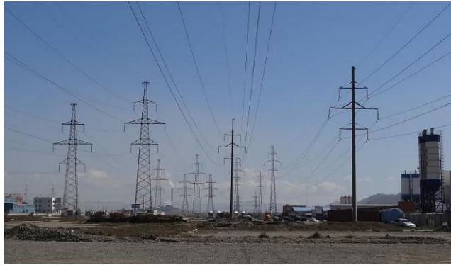
Figure 3-4 Overhead Transmission Lines near CHP 4
