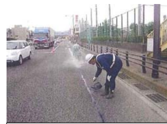
Melted asphalt into crack
