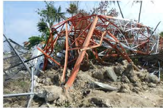
Fig. 15. Damaged tower structure flowed for about 1100 m (Balaroa).
