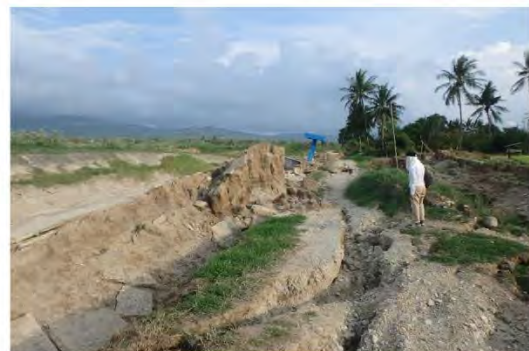
Fig. 22. Damage to irrigation channel in Jono Oge.
