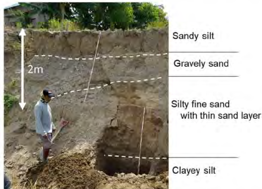
Fig. 14. Soil profile observed at the main scarp of flow-slide in Petobo.
