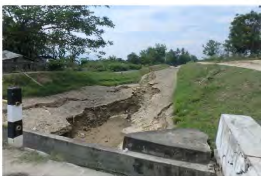
Fig. 13. Damage to the embankment of irrigation channel (Petobo).
