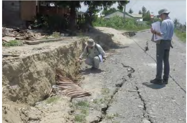
Collapse of Petobo Point Top
