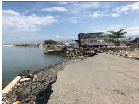
Damaged Road along Coast
