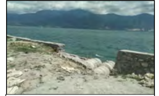
C-15. The flow of sea water broke through the gap during the tsunami
