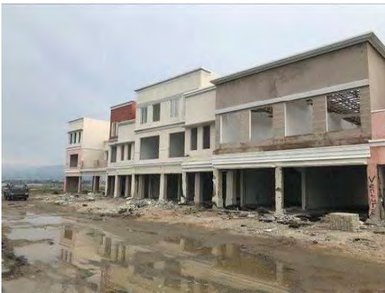
Damaged Buildings along Coast (Central East Coast)
