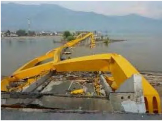
Collapsed Palu Bridge IV
