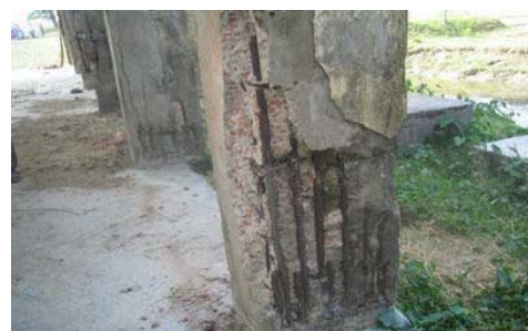
Figure-3: Column Damage by Salt Content
