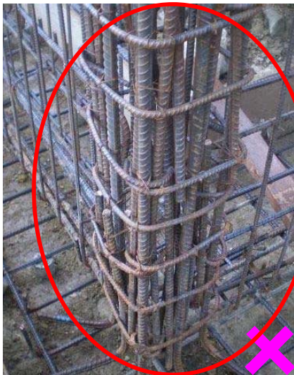
Figure-117: Wrong Bar Arrangement at Column Bottom
