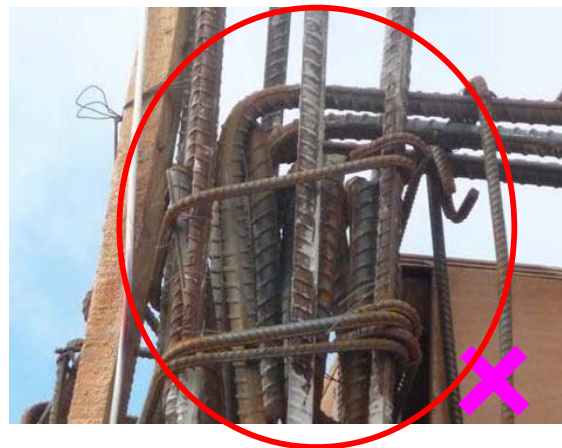
Figure-118: Wrong Bar Arrangement at Column Top
