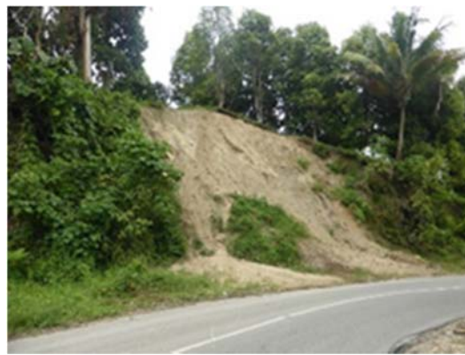
Landslides in Tompe
