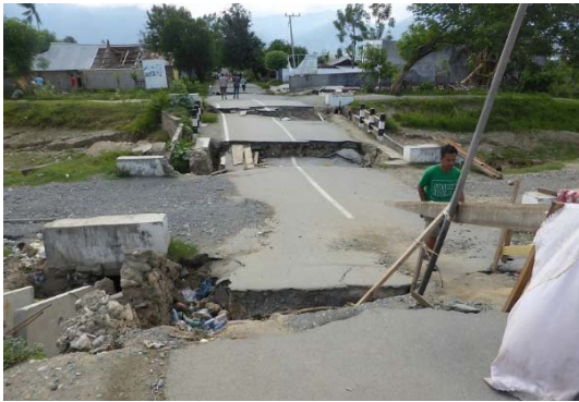
Collapse of Road near Liquefaction Area
