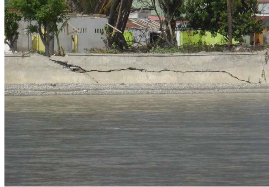
Collapse of Revetment
