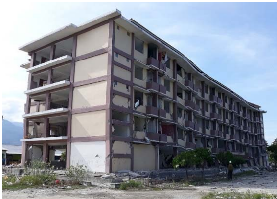
City Apartment house (Partially Damaged)
