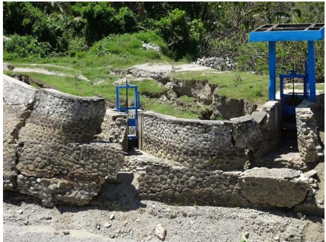
Damaged Irrigation Facilities by Ground Deformation (Watergate of Gumbasa Irrigation, Sigi Regency)
