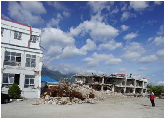
Anutapura Hospital Completely destroyed because different foundations were used on the same site
