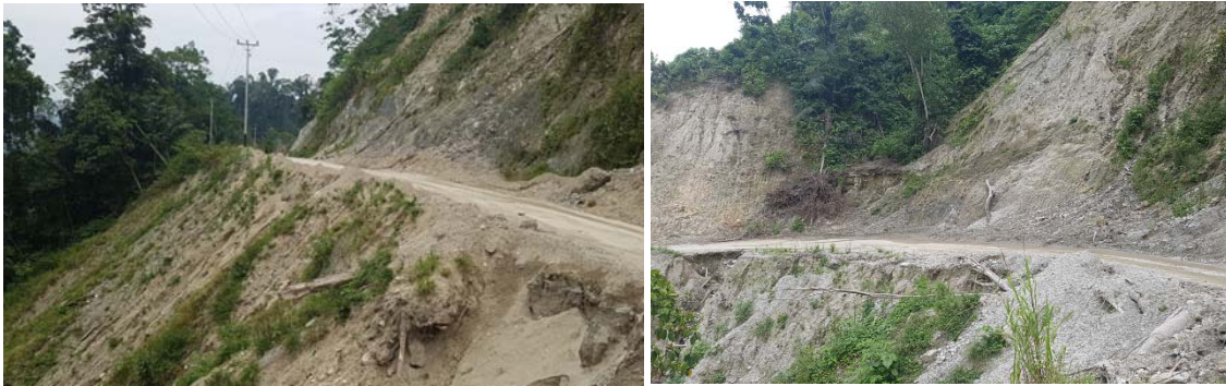
Figure 7-37 Existing Conditions (Valley side slope failure)
