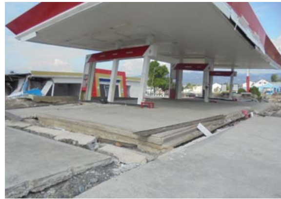
PERTAMINA Gasoline Station (Partially Damaged)
