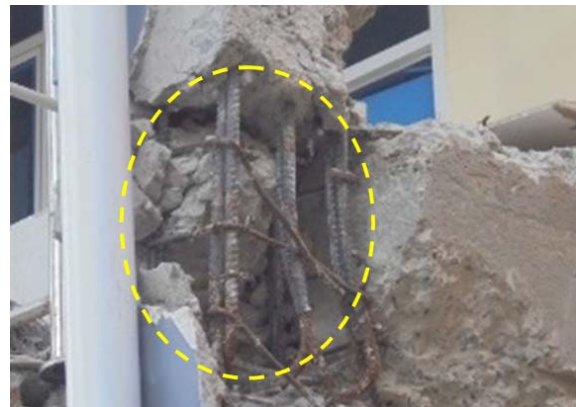
Column reinforcement exposed by the damage There was an error in the reinforcing bar arrangement in the columns
