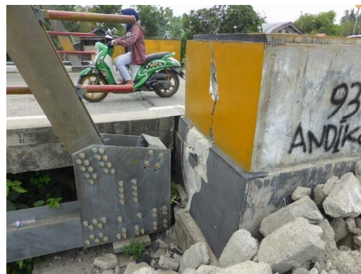
Hit of Girder on Abutment
