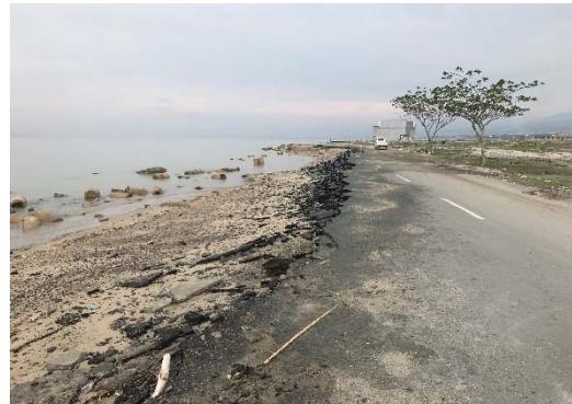
Damaged Road Surface by Tsunami
