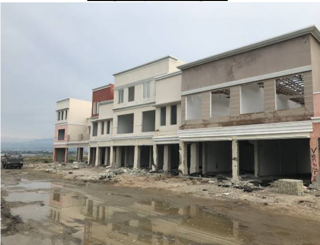
Damaged Buildings by Tsunami Inundation (100m to 450m from the Coast) (On the Right Shore of Palu Bay)
