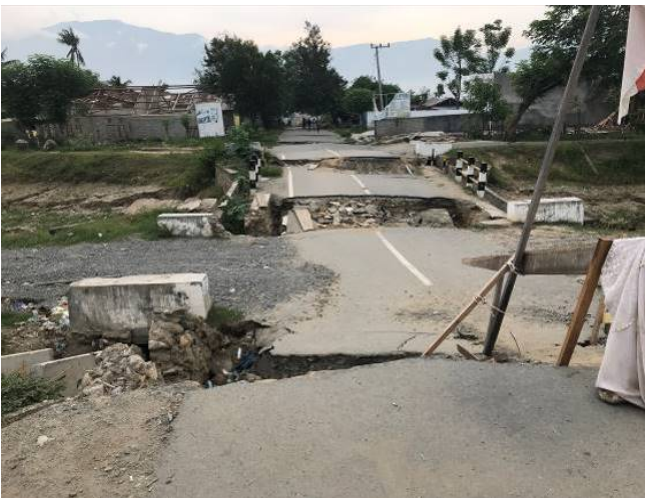
Damaged Road by Nalodo (Palu City)
