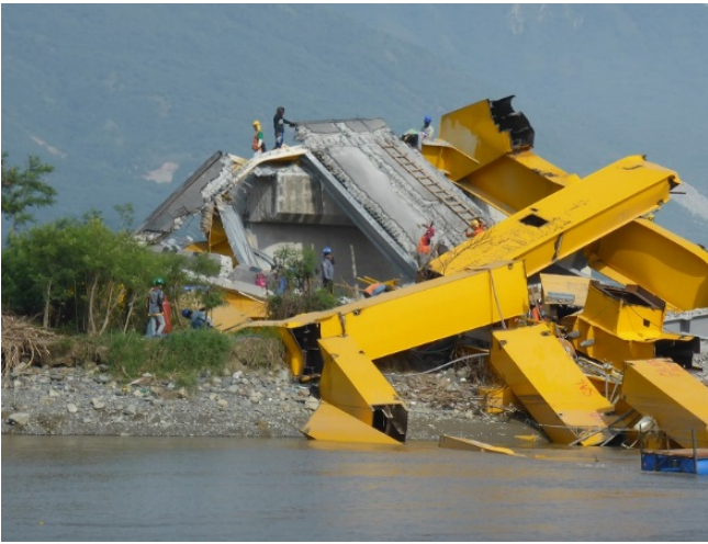
The Palu IV Bridge located at the Palu River Estuary was Collapsed by the Earthquake.
