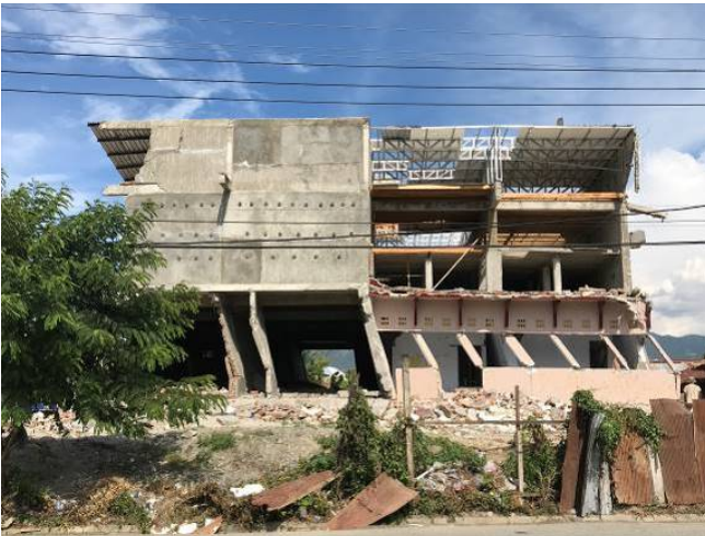
Collapsed buildings by the Earthquake (Pal City)
