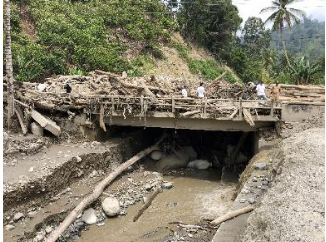
Sediment Disaster Caused by Debris Flow (Salua River, Sigi Regency)
