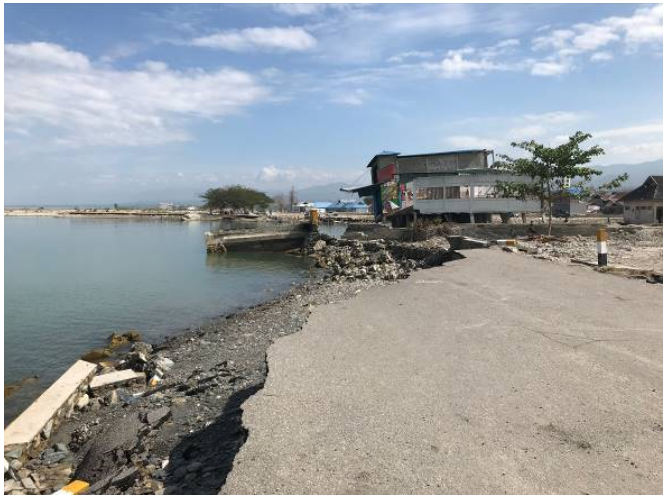
Collapsed Coastal Road along the Palu Bay
