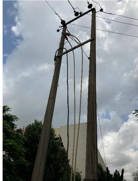
Figure 5-6.22 11kV cable discarded on site
