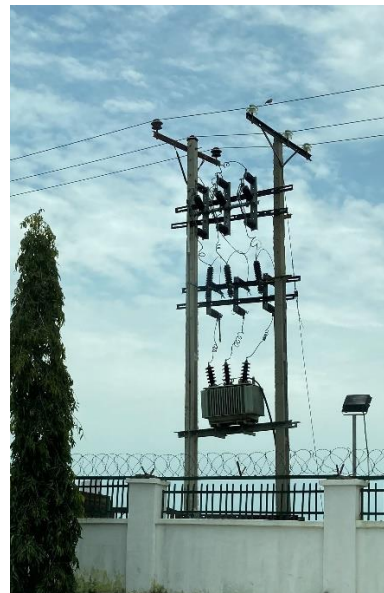
Figure 5-6.2 Pole mounted transformer
