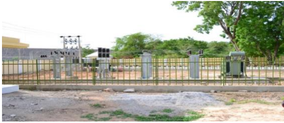
(a) 1MVA, 33kV/11kV/415V substation
