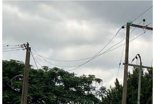
Figure 2 Large sag of conductors
