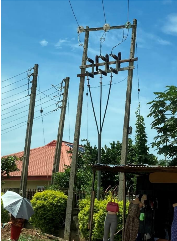
Figure 5-6.17 Poles for transformer (without arrester leads)
