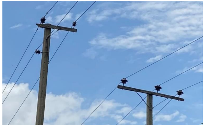
Figure 5-4.12 Broken cross arm (The right side is a 33kV line)
