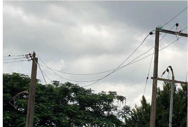
Figure 5-6.9 Large sag of conductors
