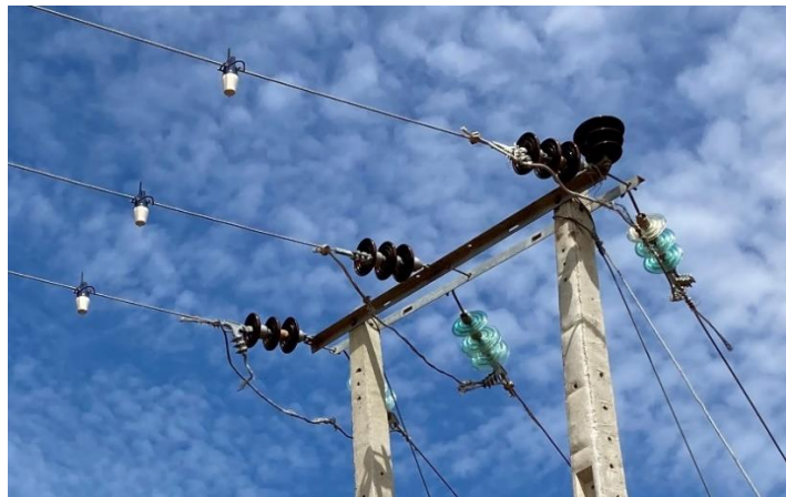
Figure 5-4.5 FCI installation status
