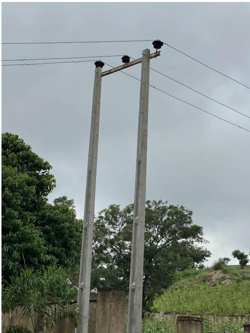
Figure 5-6.5 Square utility pole
