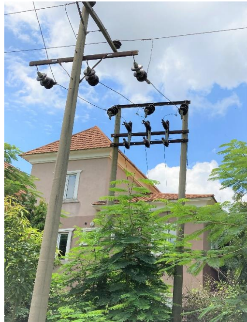
Figure 5-6.18 33kV transformer directly connected by conductor
