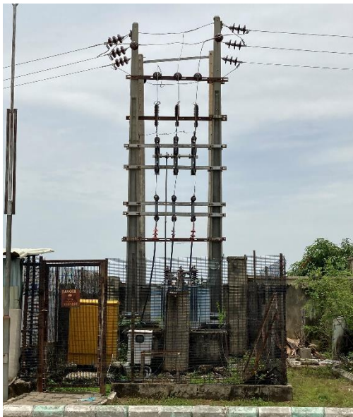
Figure 5-6.1 Ground-mounted transformer pole
