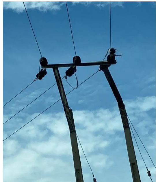
Figure 5-6.11 Broken angle for prolonging pole
