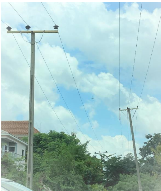
Figure 5-6.19 Inclination of 11kV pole to the 33kV line side
