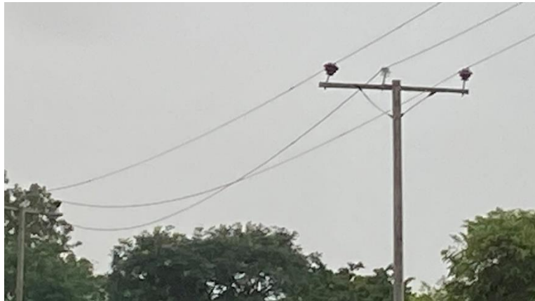
Figure 5-6.16 Large sag conductors and tilted insulators
