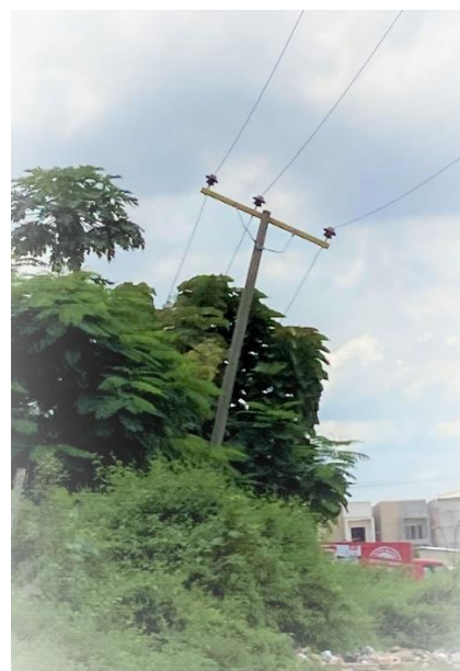
Figure 5-6.20 Inclination of 33kV pole
