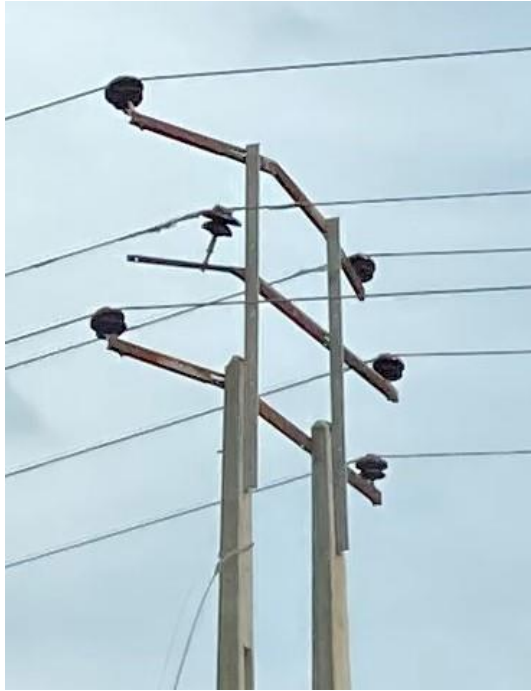
Figure 5-6.12 Arms bent ▪ Insulator detached from arm
