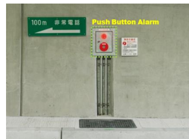
Push Button Alarm
