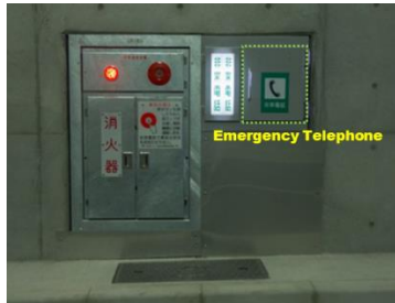
Emergency Telephone on wall
