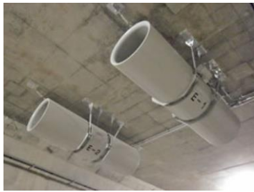
Smoke Removal System (Jet Fan)
