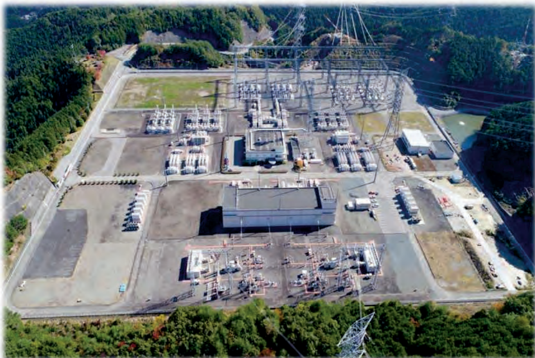
Kihoku Converter Station
