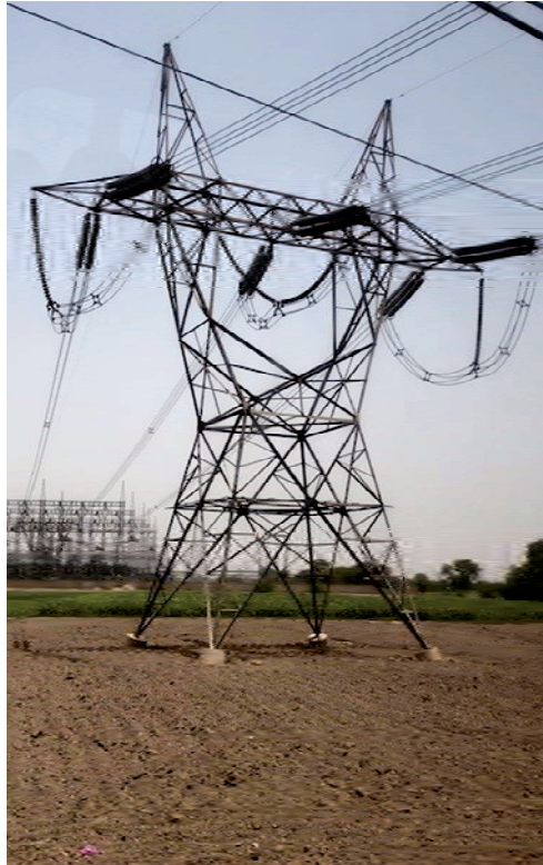
500kV Steel tower
