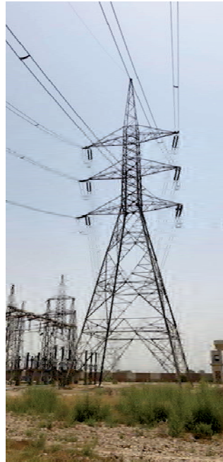
220kV Steel tower
