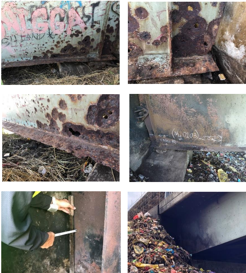
Figure 2.66 Corrosion Damages Observed
