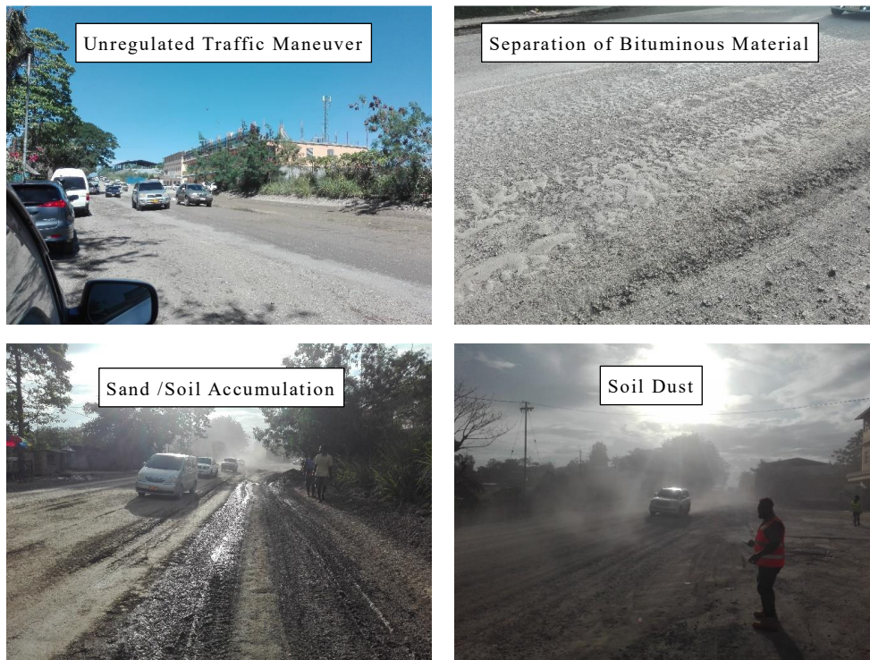
Figure 2.10 Current Condition after Rainfall
