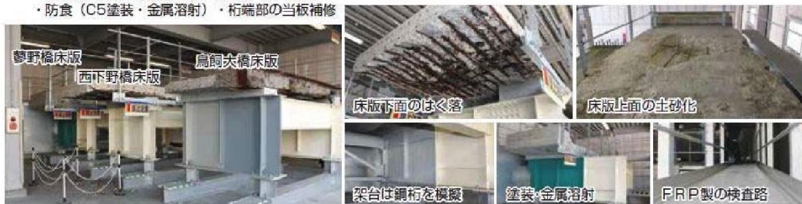
Figure 4.9 Status outside the building (Replaced bridge slab, etc.) 19
