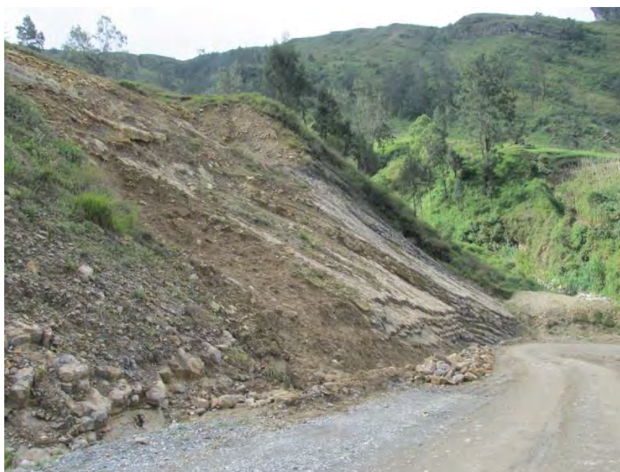
Figure 6 — Collapse due to the cut slope
