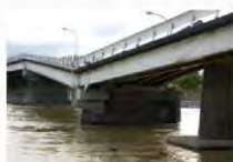
Figure 5. Bridge settlement damage due to bridge pier scouring (Japan Example)
