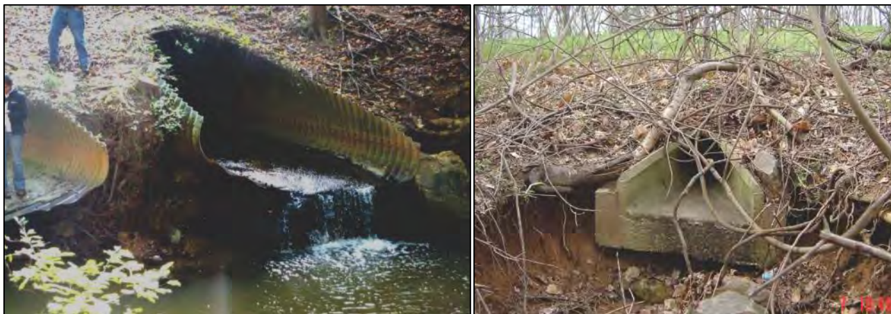
Figure 9.1 — Examples of erosion at culvert outlets (7)
