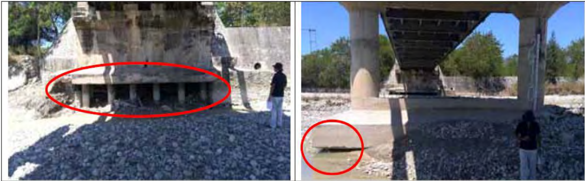
Photo Situation of damaged abutment and pier
