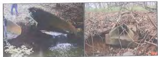
Figure 9.1 — Examples of erosion at culvert outlets (7)
