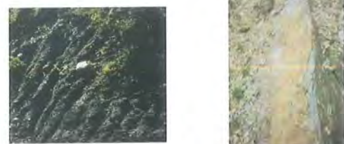
Figure 8.4 Erosion and weathering on the cut slope
