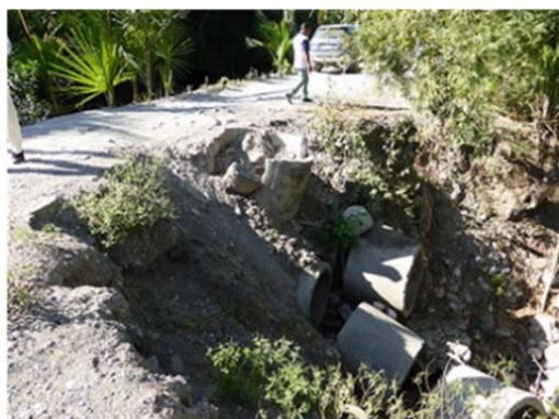
A05 Road structure damage (Sesurai)
