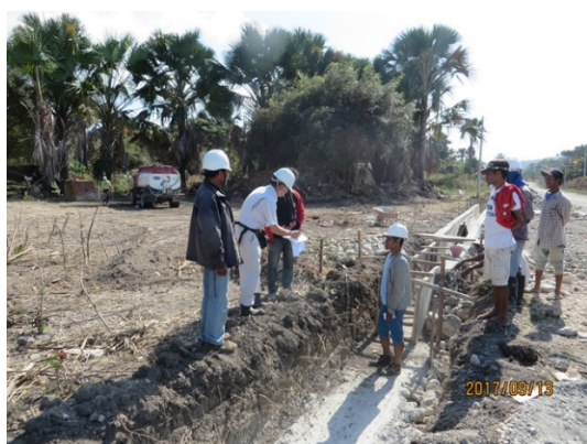
OJT for quality control of drainage on Betano-Dotic site on A14 road (No.4 of 9 Packages, 30 September, 2017)
