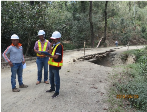
On-the-job training using checklists for cross drainage on Humboe–Letefoho emergency repair work (28 June, 2018)
