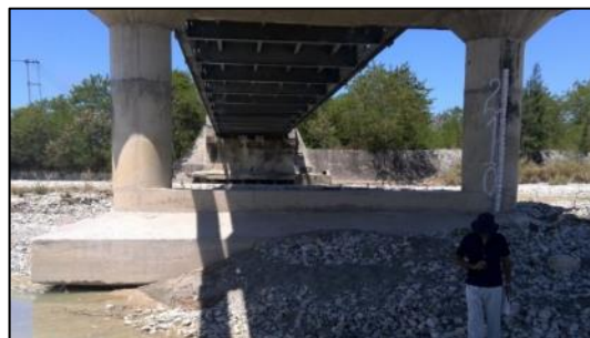
Bridge pier scouring damage (Sahen Bridge)
