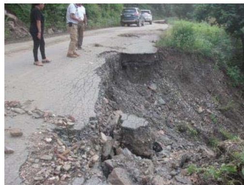
A03 Road structure damage (Likisá)
