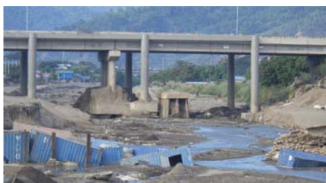
Damage of existing bridge substructure
