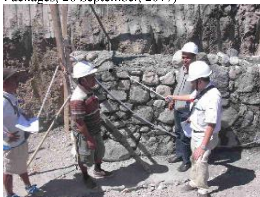
OJT for quality control of retaining walls on Ainaru-Hatudo site on C23a road (No.5 of 7 Packages, 21 August, 2017)
