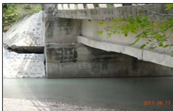
Scouring under abutment (Kelan Bridge)
