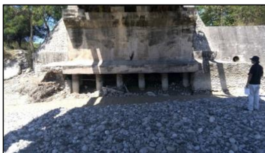
Abutment scouring damage (Sahen Bridge)
