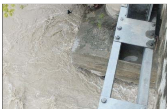
Scouring under pier (Sarai Bridge)
