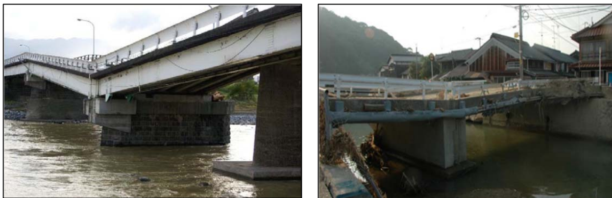
Figure 2.25 Example of damage due to scouring (Japan)
