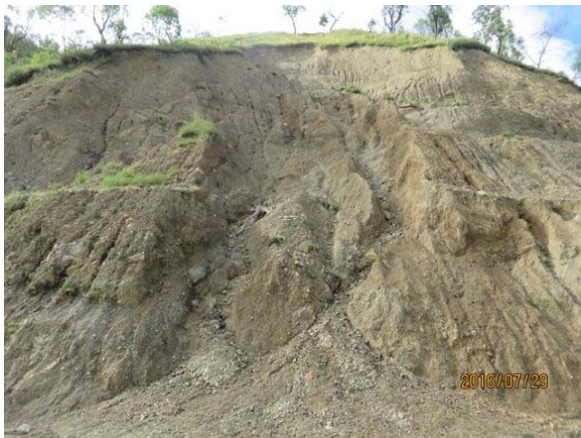
Surface layer collapse
