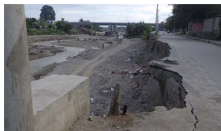
Retaining wall damage
