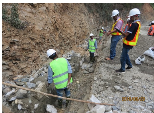
On-the-job training using checklists for masonry retaining walls on Humboe–Letefoho emergency repair work (28 June, 2018)
