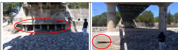
Photo2.1 Situation of Damaged Abutment and Pier
