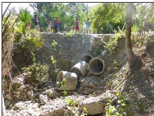
Damaged road and culvert (Sesurai culvert)
