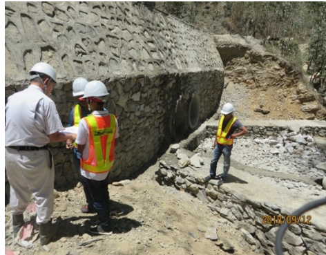
On-the-job training using checklists for cross drainage on Humboe–Letefoho emergency repair work (12 September, 2018)
