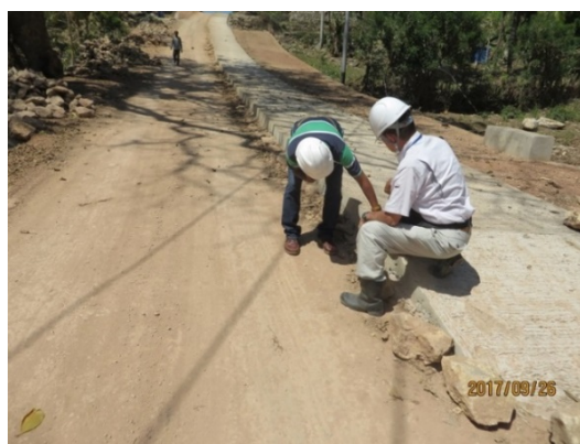
OJT for quality control of concrete pavement on Iliomar and Lospalos sites on A08 road (No.1 of 9 Packages, 26 September, 2017)
