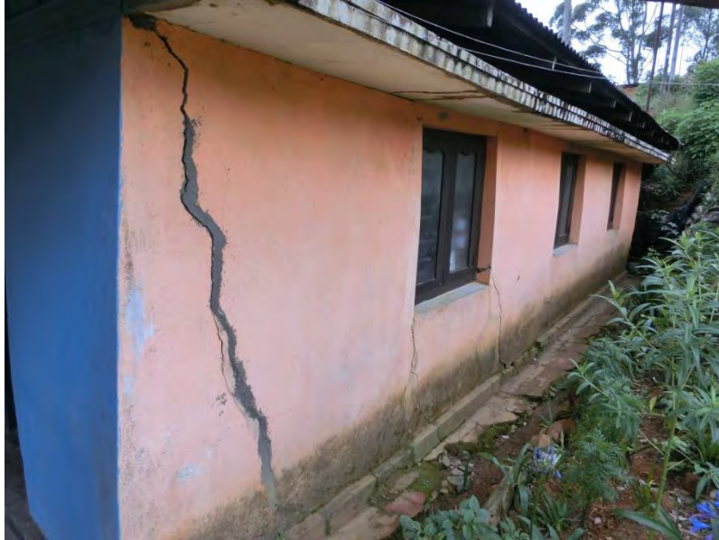
Figure 3 — Crack at the house near Landslide area (Landslide in Sri Lanka)
