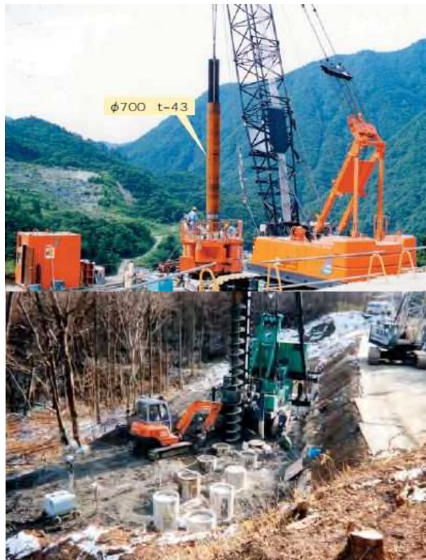
Photo. 4.2 Execution of pile work of steel pipe for mass movement prevention in Japan
