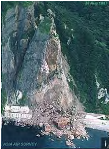
T3 Rock mass failure
