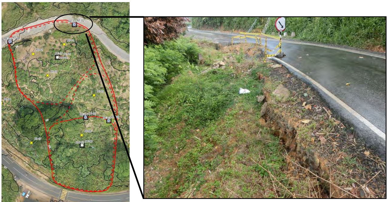
Figure 2 — Crack in the road surface and shoulder (Landslide in Sri Lanka)
