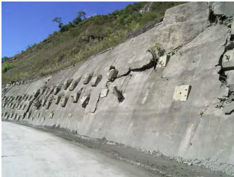
Photo.1.1 Failure example of mass movement countermeasure
