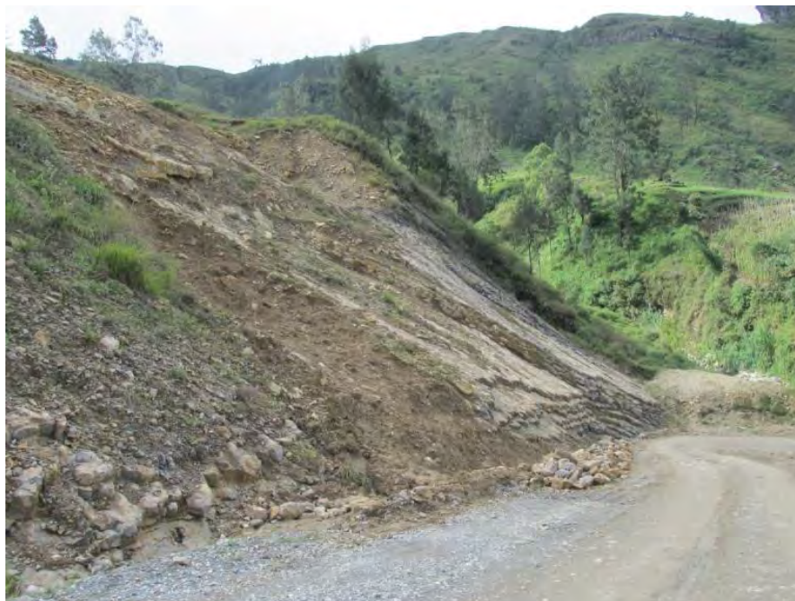
Figure 6 — Collapse due to the cut slope
