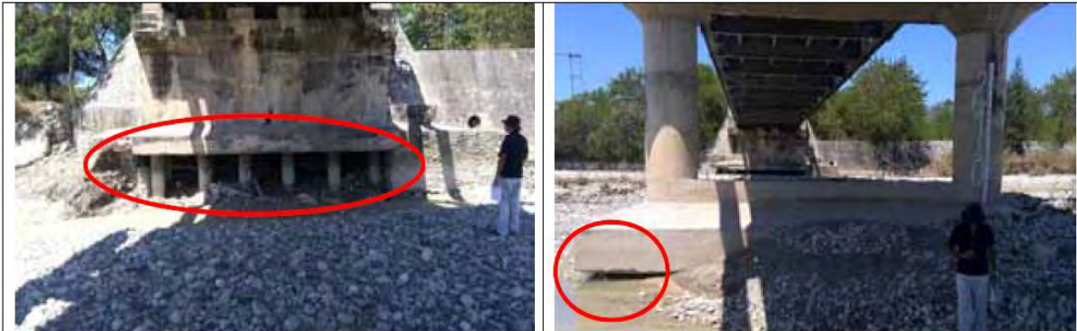
Photo Situation of damaged abutment and pier
