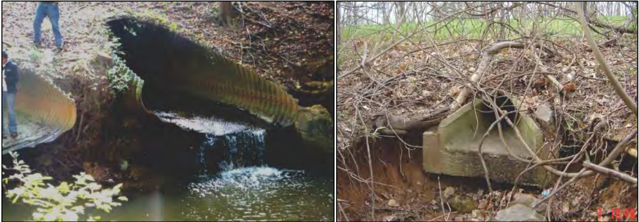
Figure 9.1 — Examples of erosion at culvert outlets (7)
