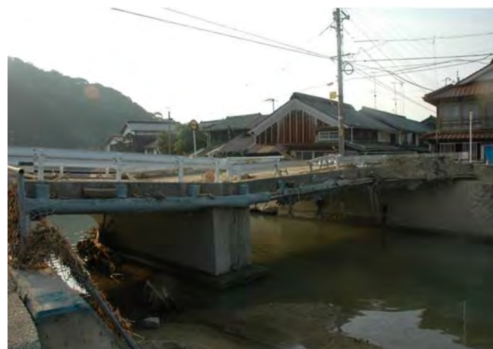
Figure 7 — Bridge settlement damage due to bridge pier scouring (Japan example)
