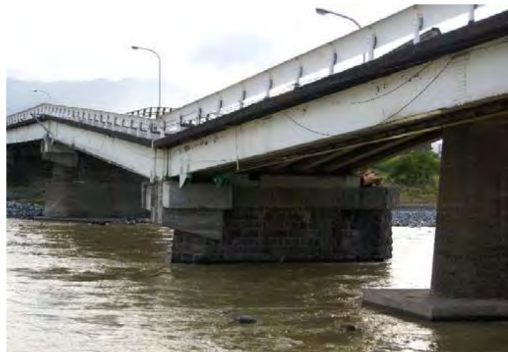
Figure 6 — Bridge settlement damage due to bridge pier scouring (Japan example)
