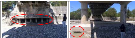
Photo2.1 Situation of Damaged Abutment and Pier
