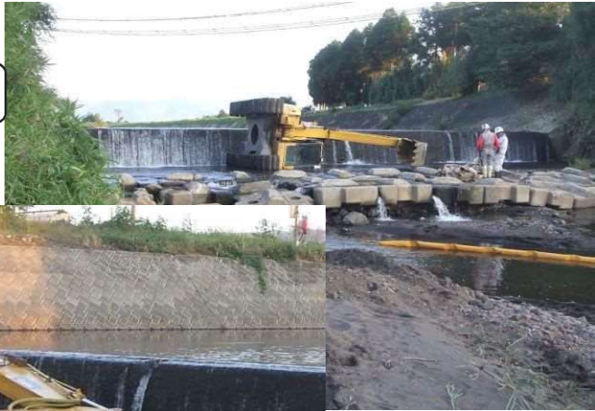
Over-turning when trying to climb up river dam
