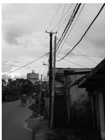
Figure 21.3.9 20kV Distribution Line
