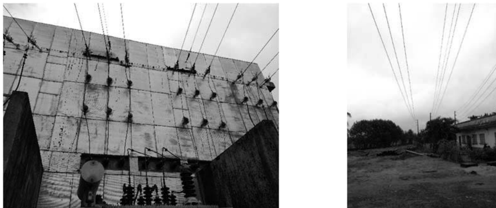
Figure 21.3.8 Existing 35 kV Transmission Line
