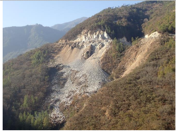
Photo 2: Slope failure along the road from Paro to Haa
