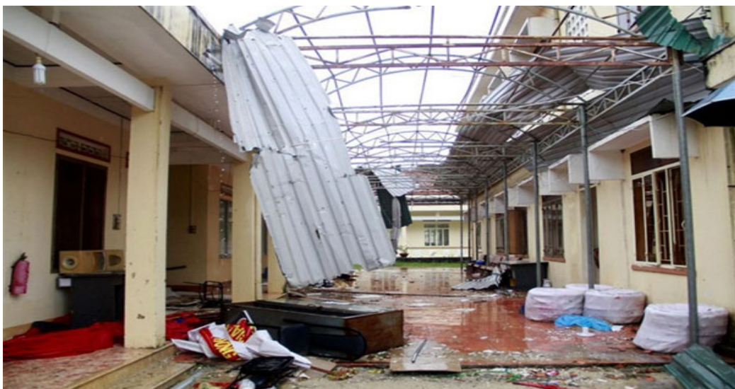
Photo 2. Hospital facilities are seriously damaged by the typhoon
