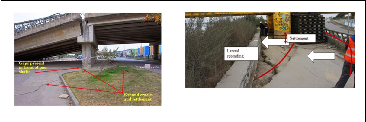
Figure 2.2-3 Damages caused by Liquefaction
