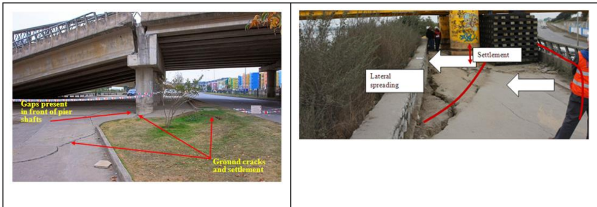
Figure 8.4-2 Damages caused by Liquefaction
