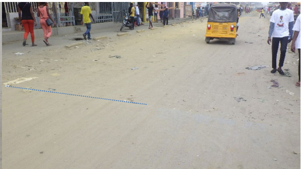
Destructed existing pavement due to high groundwater level
