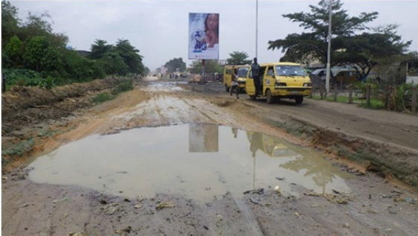
Water ponding in the existing road at around PK2.0 km
