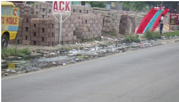
Non-functional existing side ditch by the improper slope gradient at PK1.2 km RHS
