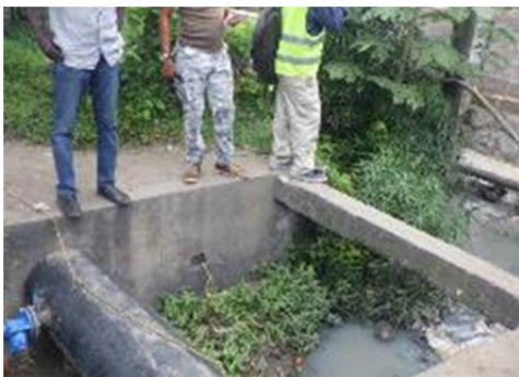
FD500mm and AC100mm Appeared on RHS at PK0.65 km on 16 November 2018
