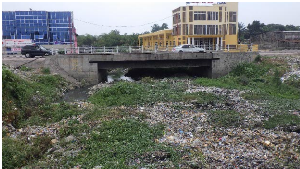
Bridge over Yolo River Crossing at Lumumba Road located downstream from University Avenue observed on 14 Oct. 2018
