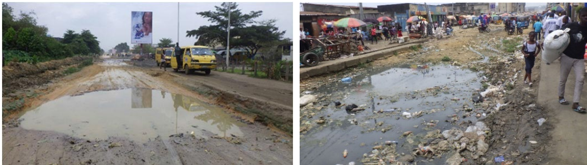
Water ponding in the existing road at around PK2.0 km
