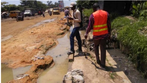
Blocked ditch (on the right)
