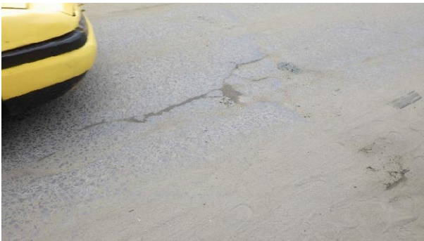
Cracks due to high groundwater level around PK5.5 km
