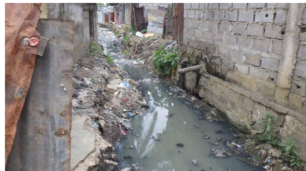
Downstream (3.0 m width and 1.0 m depth on average) between buildings at PK3.95 km
