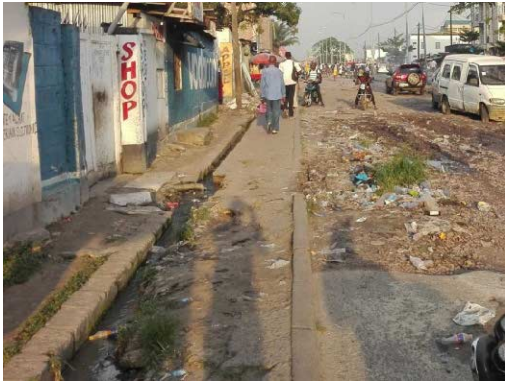
Deteriorated pedestrian pavement, Avenue Bongolo
