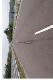
Figure 6.15 Cracks Observed on the Deck of the N'SELE Bridge on National Route 1
