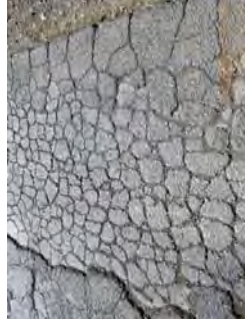
Figure 6.14 Generalized Cracks/Alligator cracks
