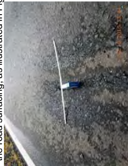
Figure 6.6 Road Settling /Hollow
