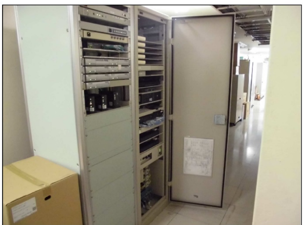
CCTV Central Equipment (uncovered)
