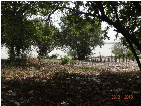
Photo: The Area near Monkey Point Tide Gauge after the Tide Gauge was collapsed
