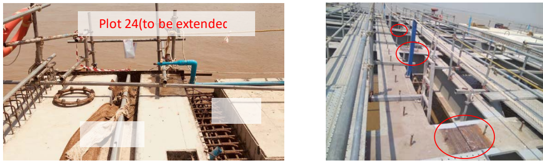
a) Rail trench at Plot 25 to be extended continuously to Plot 24 b) Rigid connection between blocks by welding (11 locations in cross-section direction)
