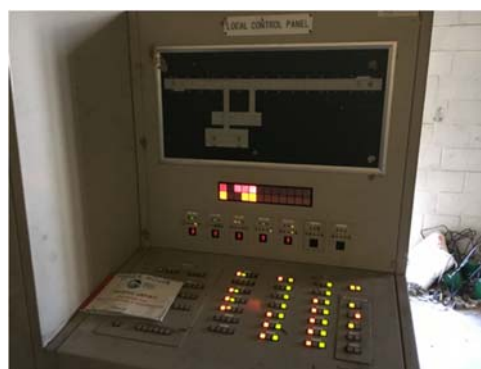
Photo 24 Lights Control Panel in power room 1F
