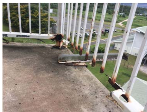
Photo 16 Rusted Steel fence
