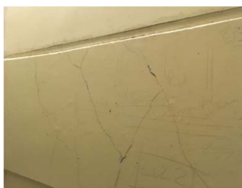
Photo 18 Cracks on pillar and Beam
