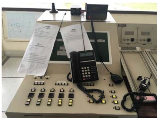
Photo 23 Failed Lights Control Panel in ATC
