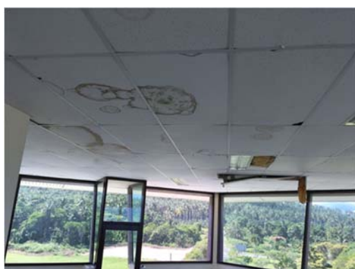
Photo 17 Remarkable Leaking in Control Cabin
