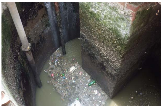
Inlet Chamber and Suction Pipe
