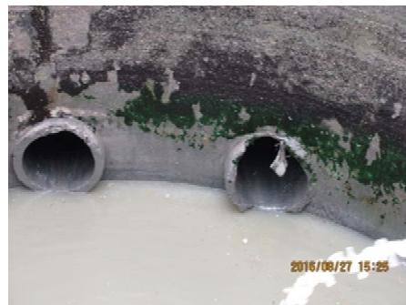
Inlet Pipes and Pump Well
