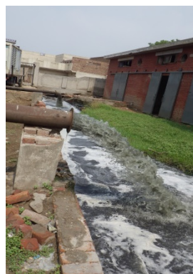
Delivery Pipe and Discharge Channel
