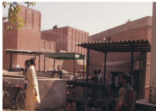
Pump Well and Pump House
