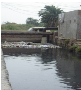
Discharge Drain – Drainage Channel No.1
