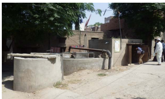
Pump Well and Pump House
