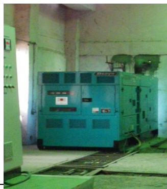
Power Receiving Equipment
