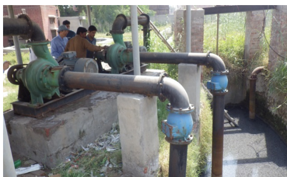
Pump Well and Suction Pipe
