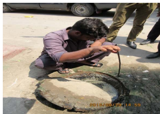
Blockage of Sewer Pipe Near WP14
