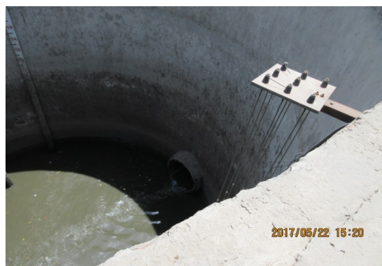
Inlet pipe and Pump Well
