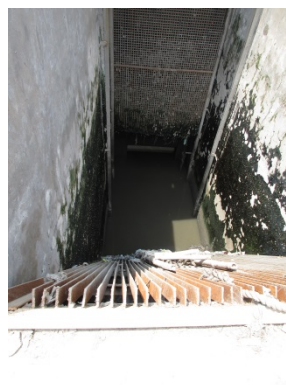
Preliminary Treatment Facility
