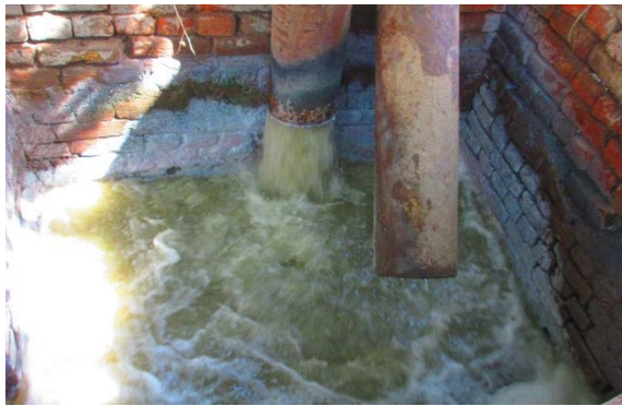
Delivery Pipe and Chamber
