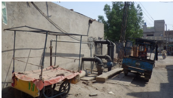
Discharge Chamber and Pipe
