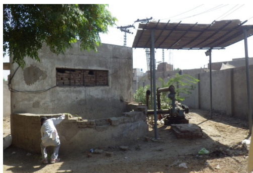
Pump Room and Pump Unit
