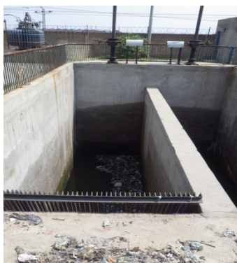
Inlet Gate and Coarse Screen
