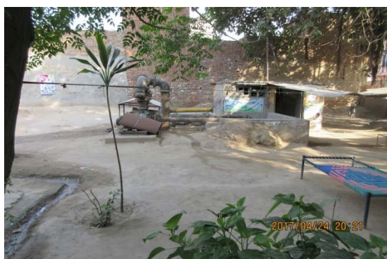
Pump Well and Pump Equipment
