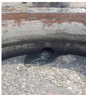
Inlet Pipe and Pump Well
