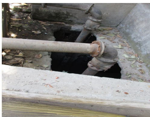
Pump Well and Suction Pipe
