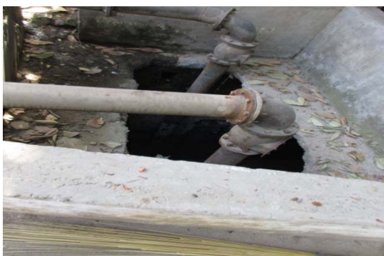
Pump Well and Suction Pipe
