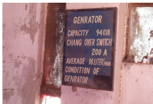
Name Plate of Generator
