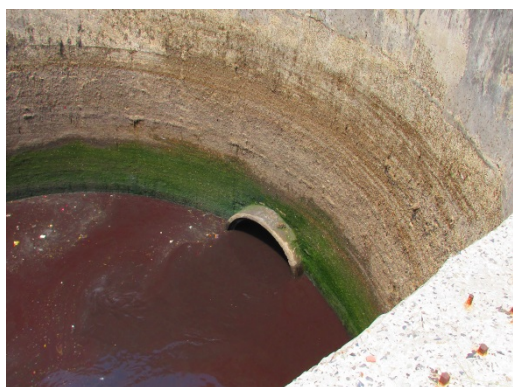
Inlet Pipe and Pump Well
