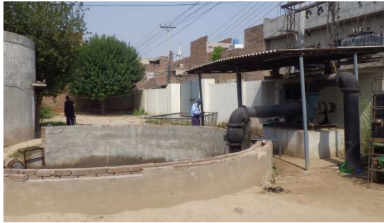
Pump Unit and Suction Pipe
