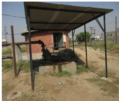
Pump Room and Pump Unit
