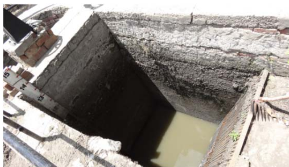
Preliminary Treatment Facility
