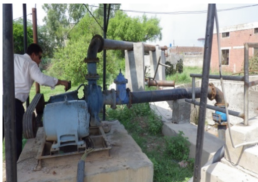
Suction and Delivery Pipe
