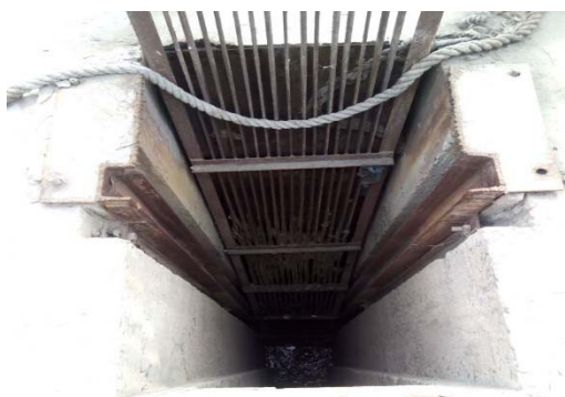
Receiving and Flow Adjustment Well
