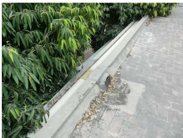
Water collector pipe and intake port
