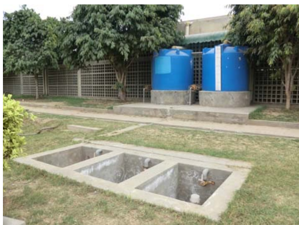
Tanks and concrete pits
