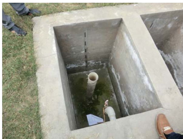
Recharge well in concrete pit
