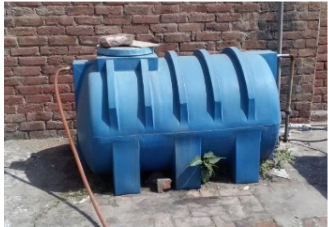
Tank for storing discharged water from Well
