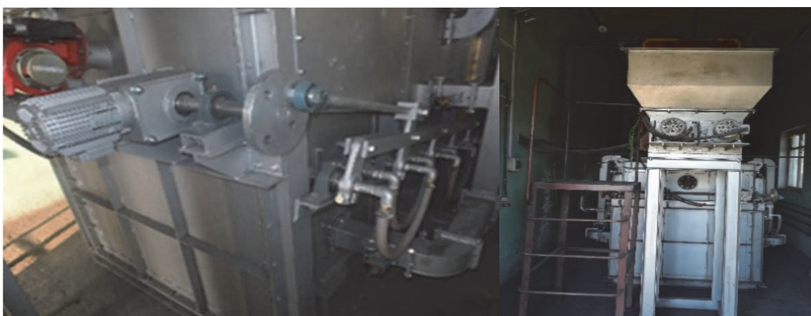
Heat Only Boiler (HOB) Existing MUHT-3
