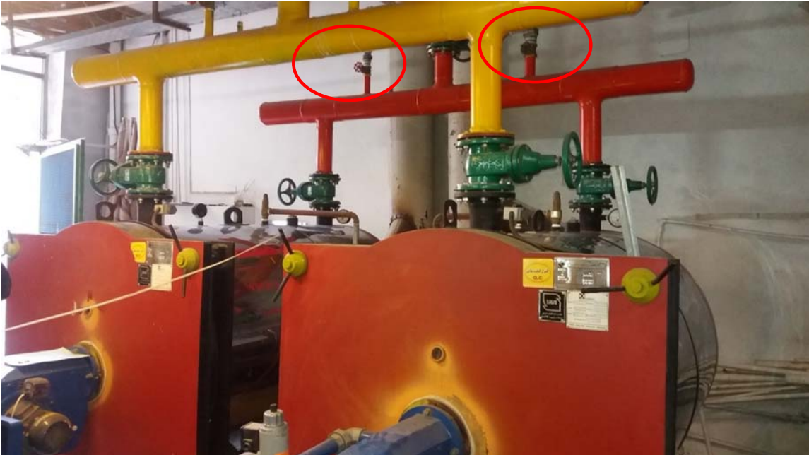
Fig. 6: Valve in the direction of the pipe connection of the expansion vessel to the boilers
